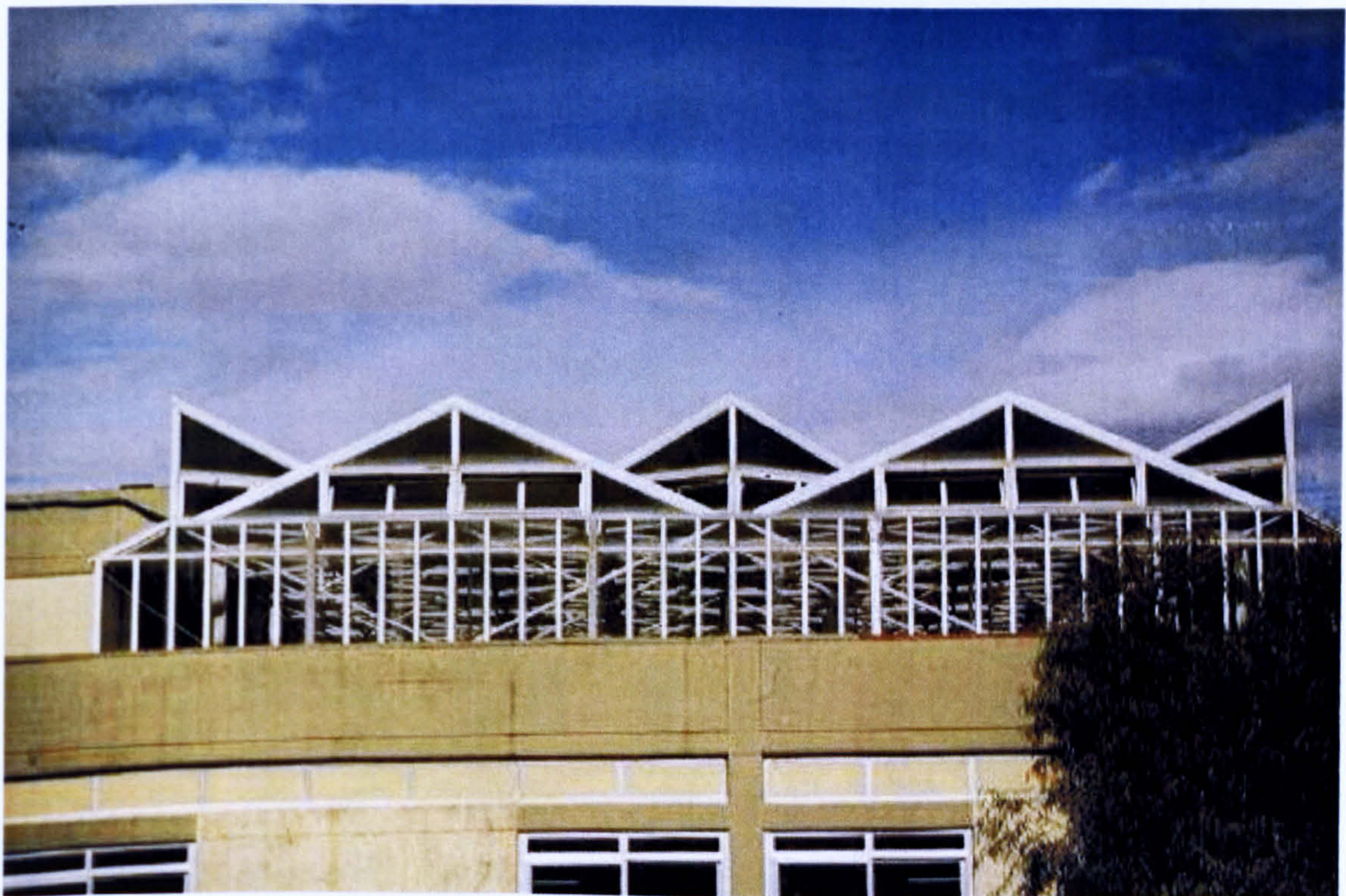
Figure 4. 5: The solar roof from the South
