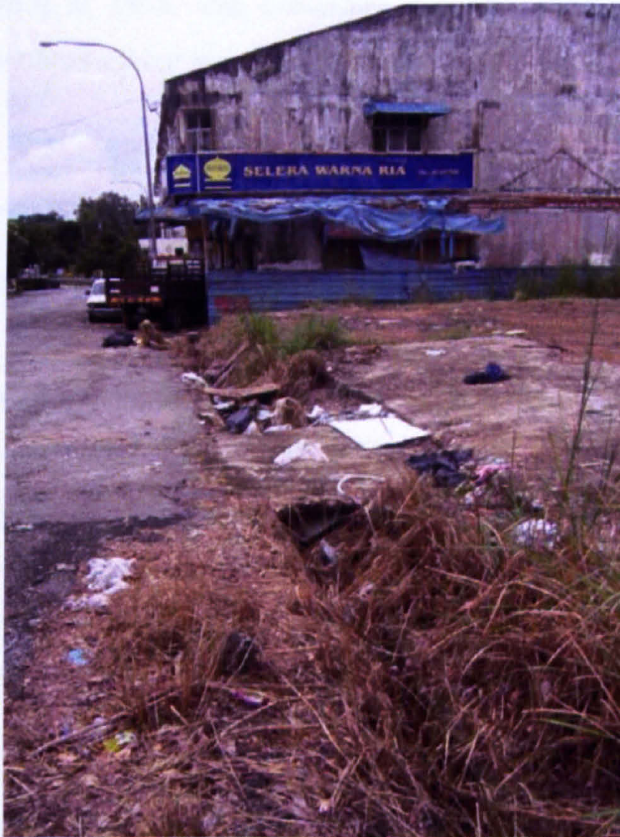
Figure 5.1.2: Poor maintenance of drains in a residential area in JB.
