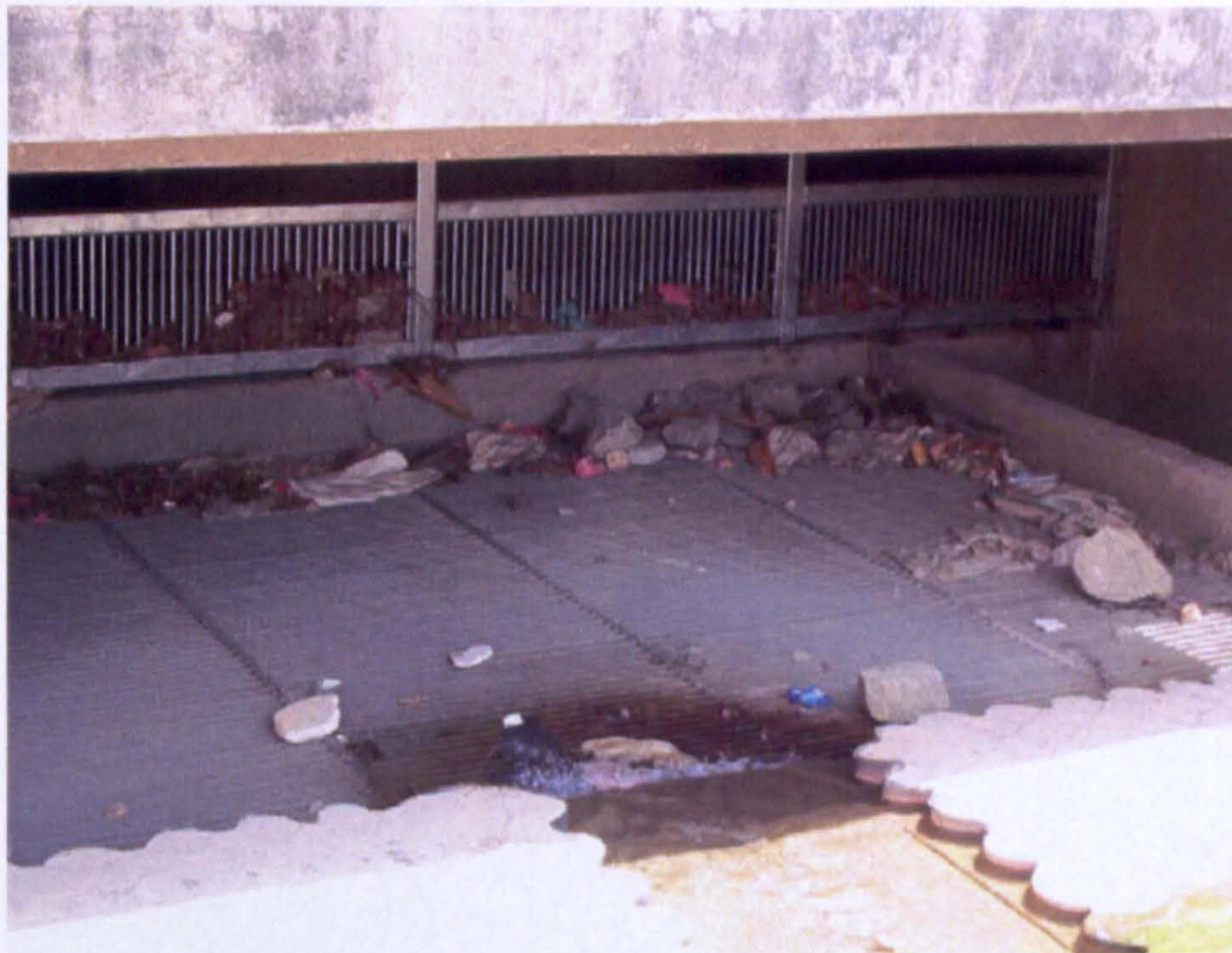
Figure 5.2.10: Solid waste traps on the GPT will be cleaned by maintenance workers.
