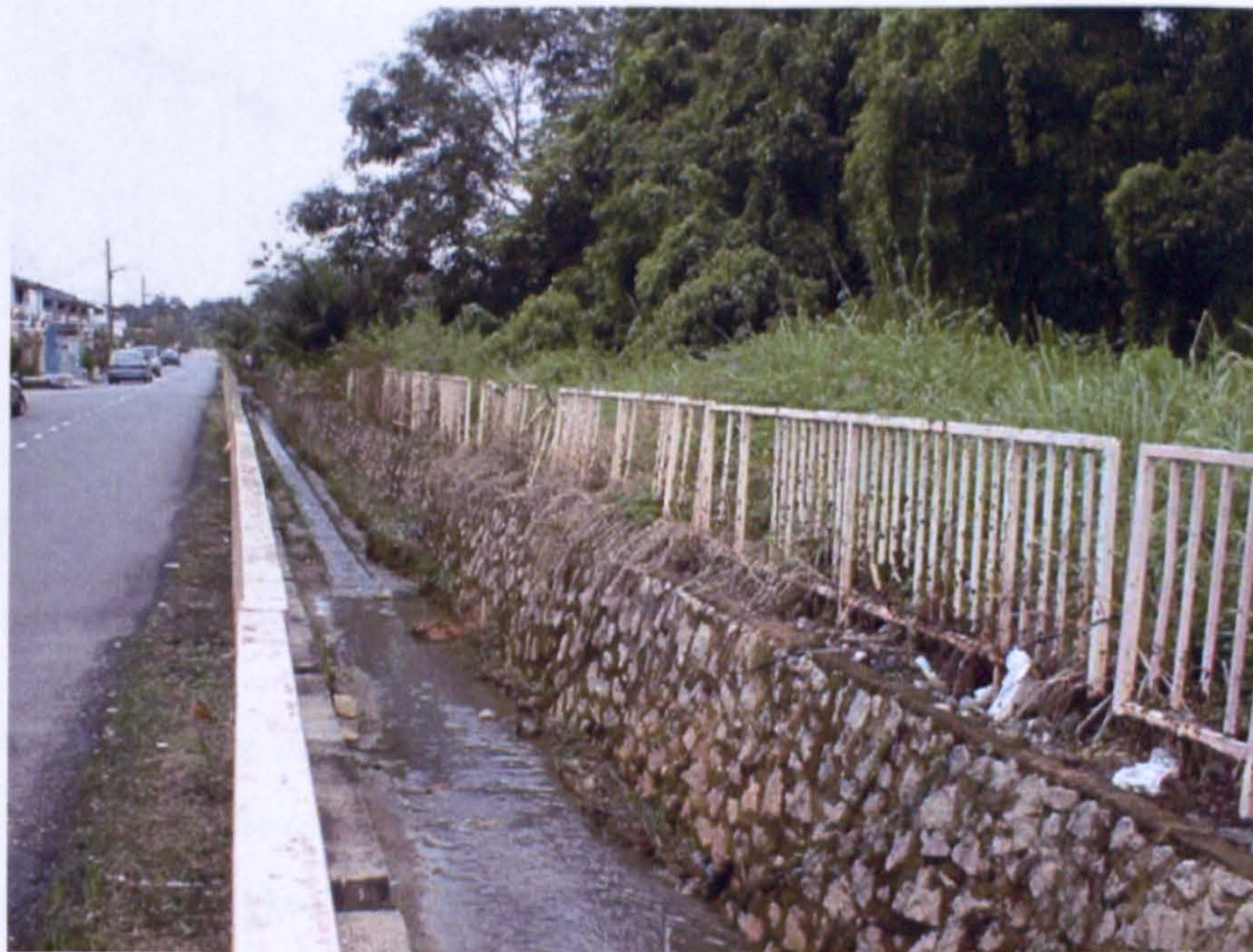
Figure 5.1.8: A damaged fence for the drainage resulting from rust in a residential area in JB.
