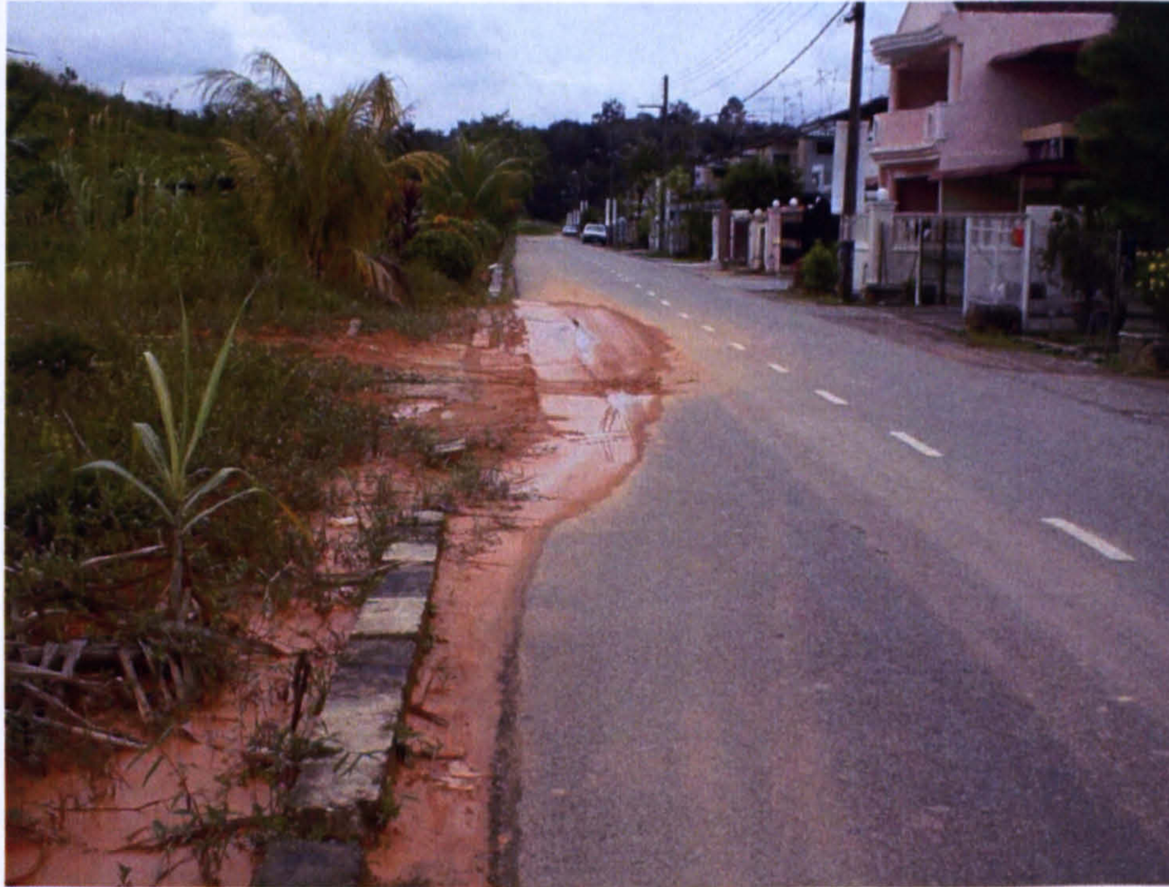
Figure 5.1.4: Siltation and blockage of the drainage system from nearby development activities in a residential area in JB.
