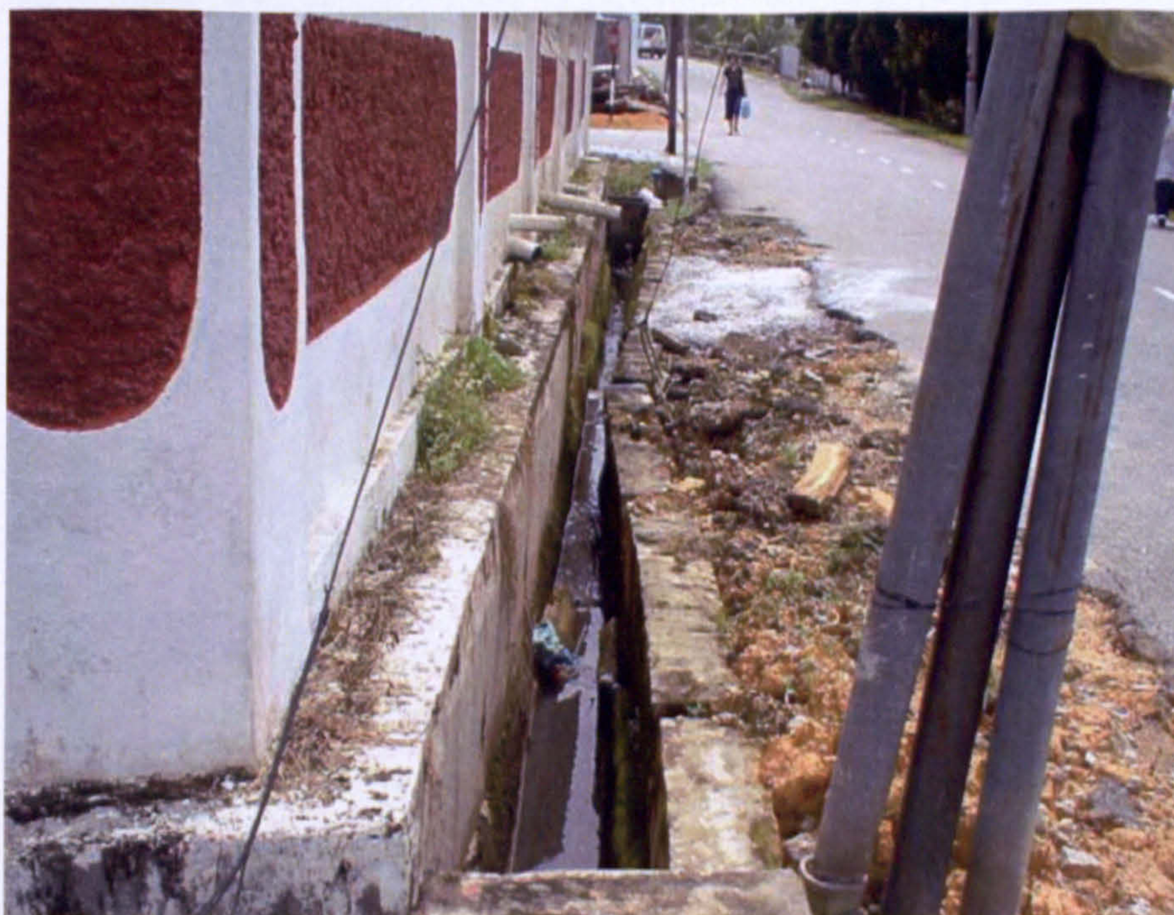
Figure 5.1.9: A collapsed drain wall in need of urgent maintenance in a residential area in JB.
