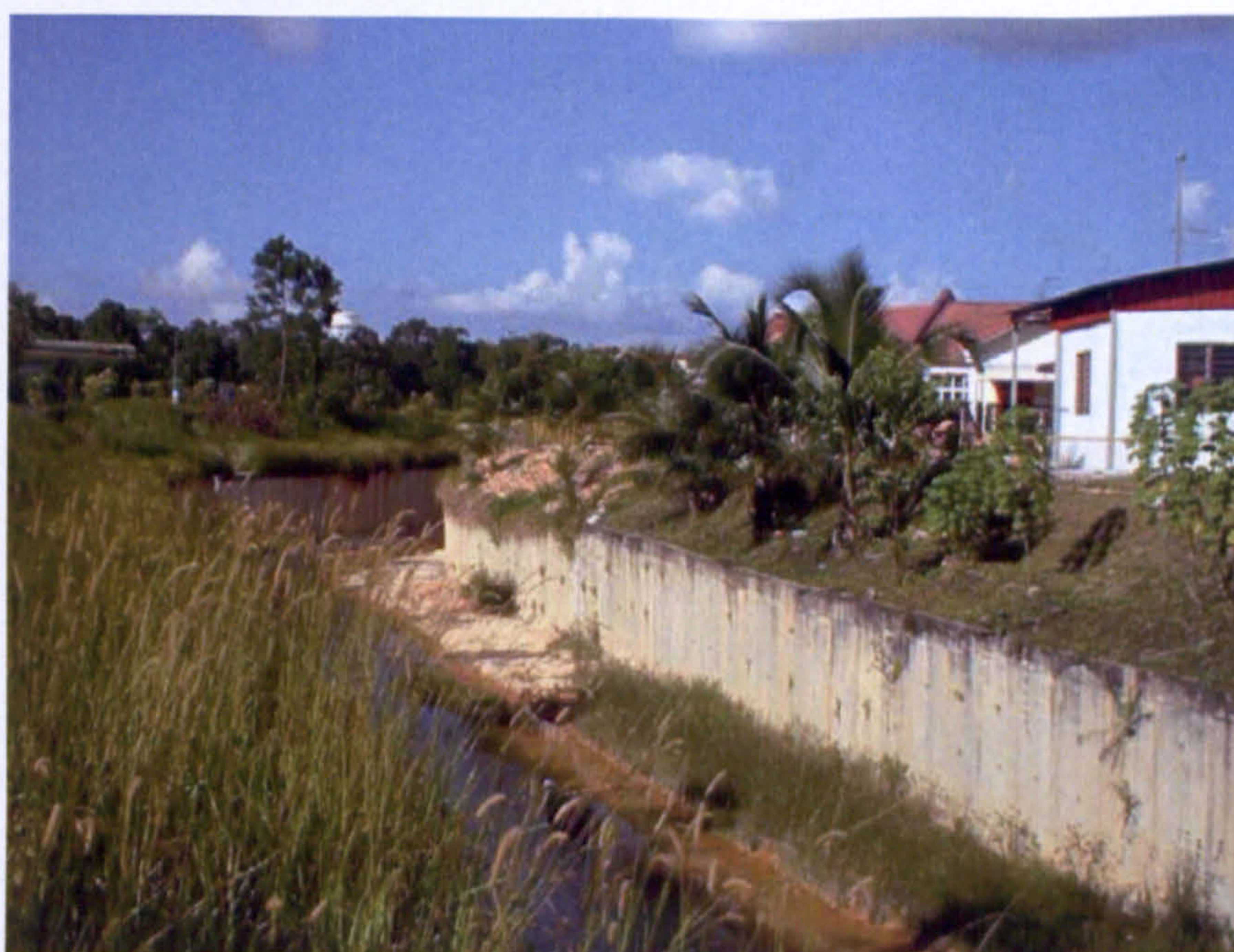
Figure 5.1.13: The storm drain is behind a house which is very dangerous especially for children.
