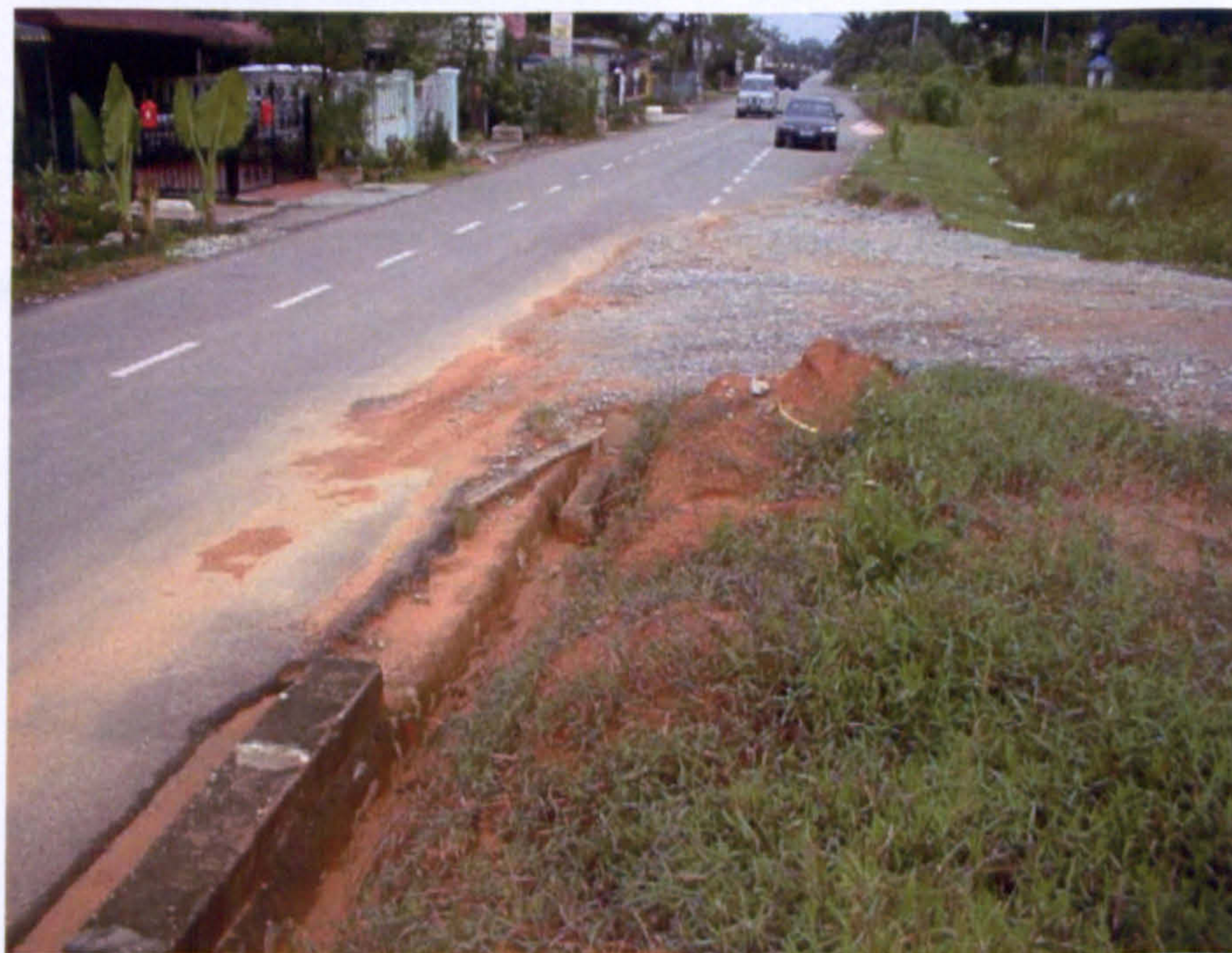
Figure 5.1.11: A drain blocked by silt from a nearby construction site. The road was also muddy.
