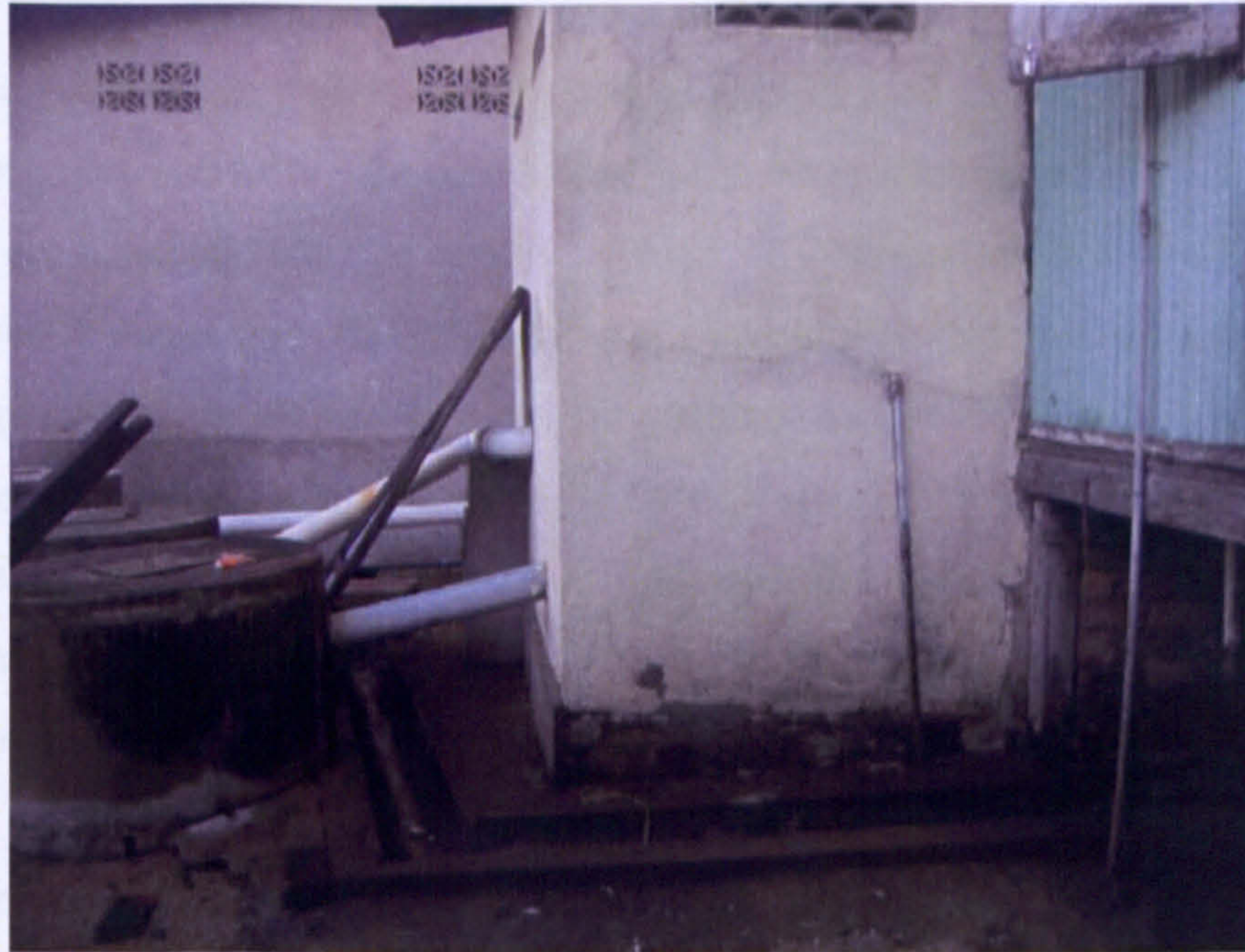
Figure 3.4.1: Toilet wastes are drained into tanks made from concrete culvert.
