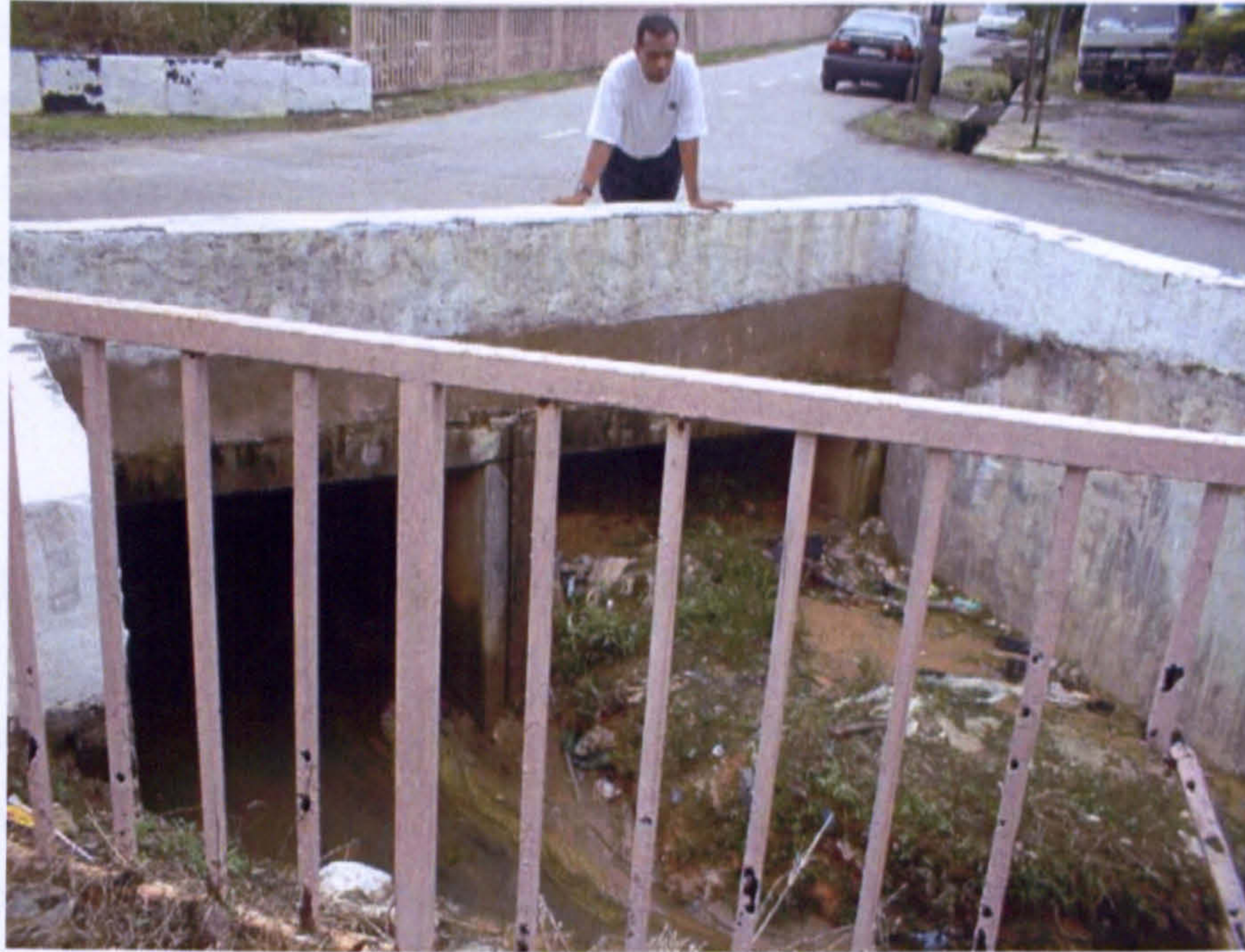
Figure 5.1.3: The drainage in residential areas needs improvement and maintenance.
