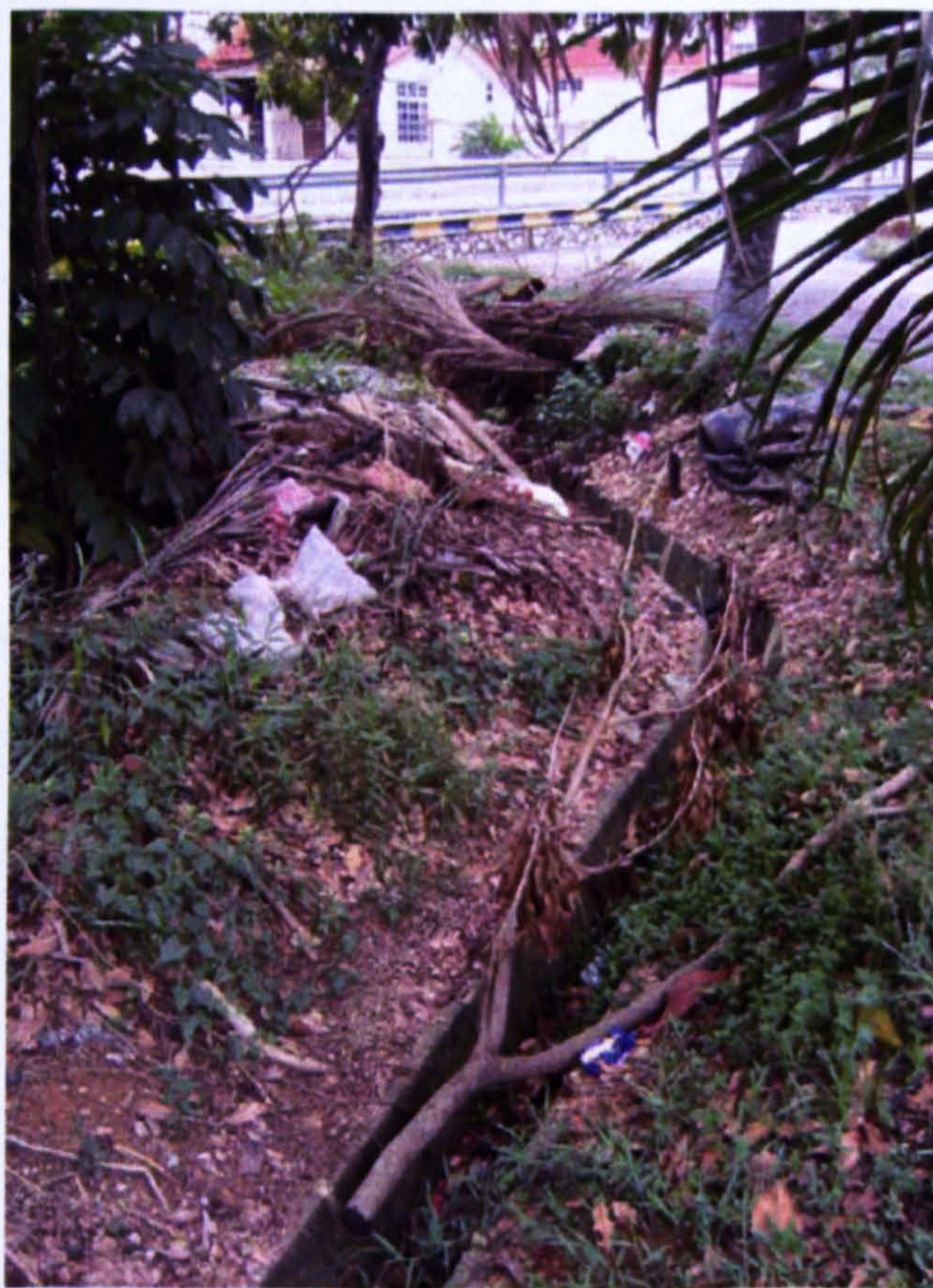
Figure 5.1.7: Drainage with improper maintenance in a JB residential area.
