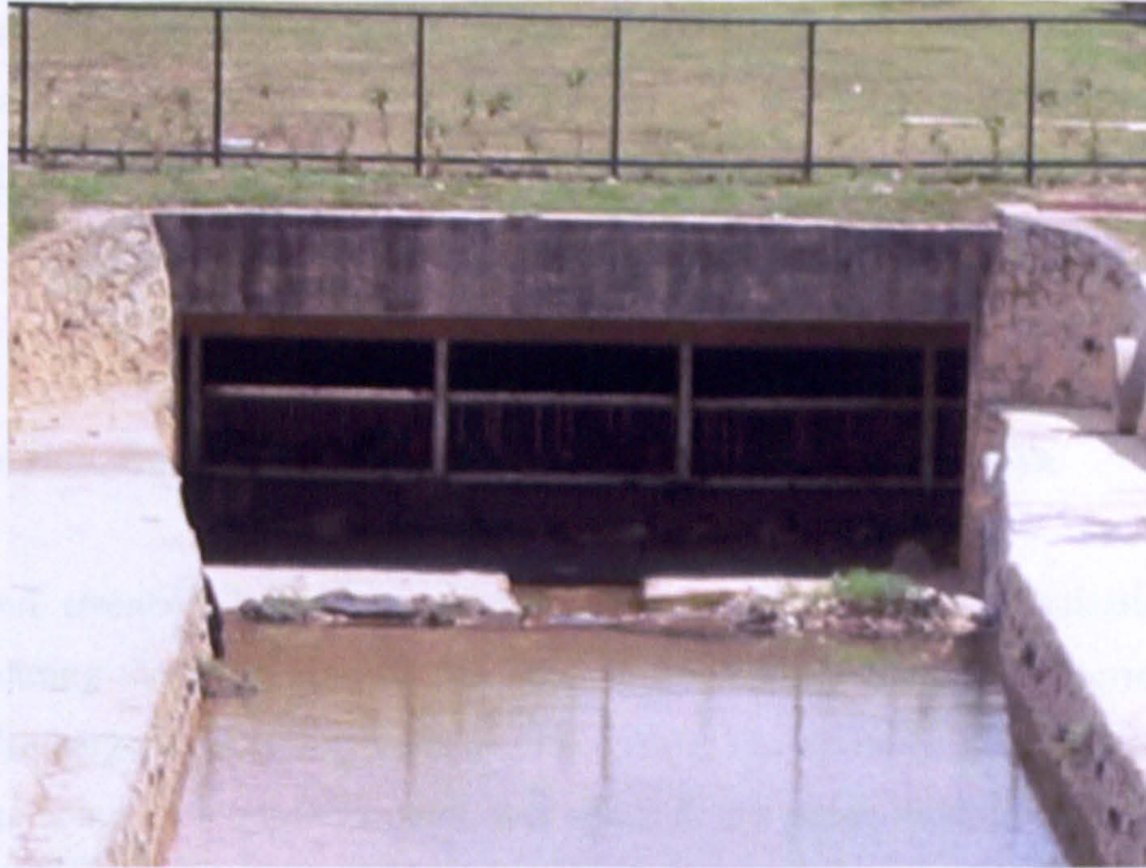
Figure 5.2.9: GPT type 3 installed in the main drain to trap solid waste.
