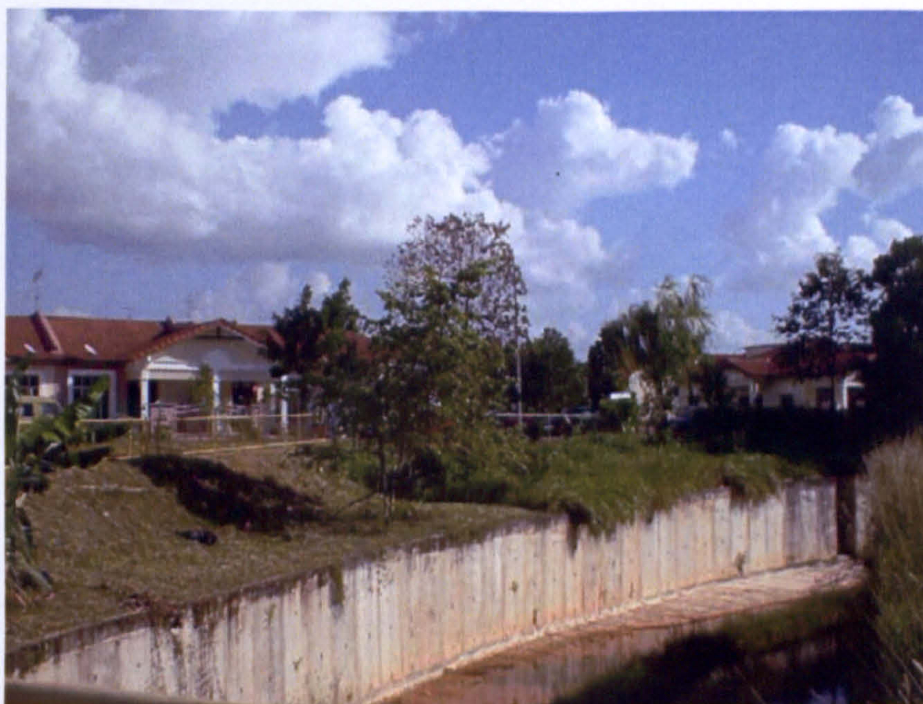
Figure 5.1.12: The distance between the residential block and the storm drain are close to each other in a residential area in JB.
