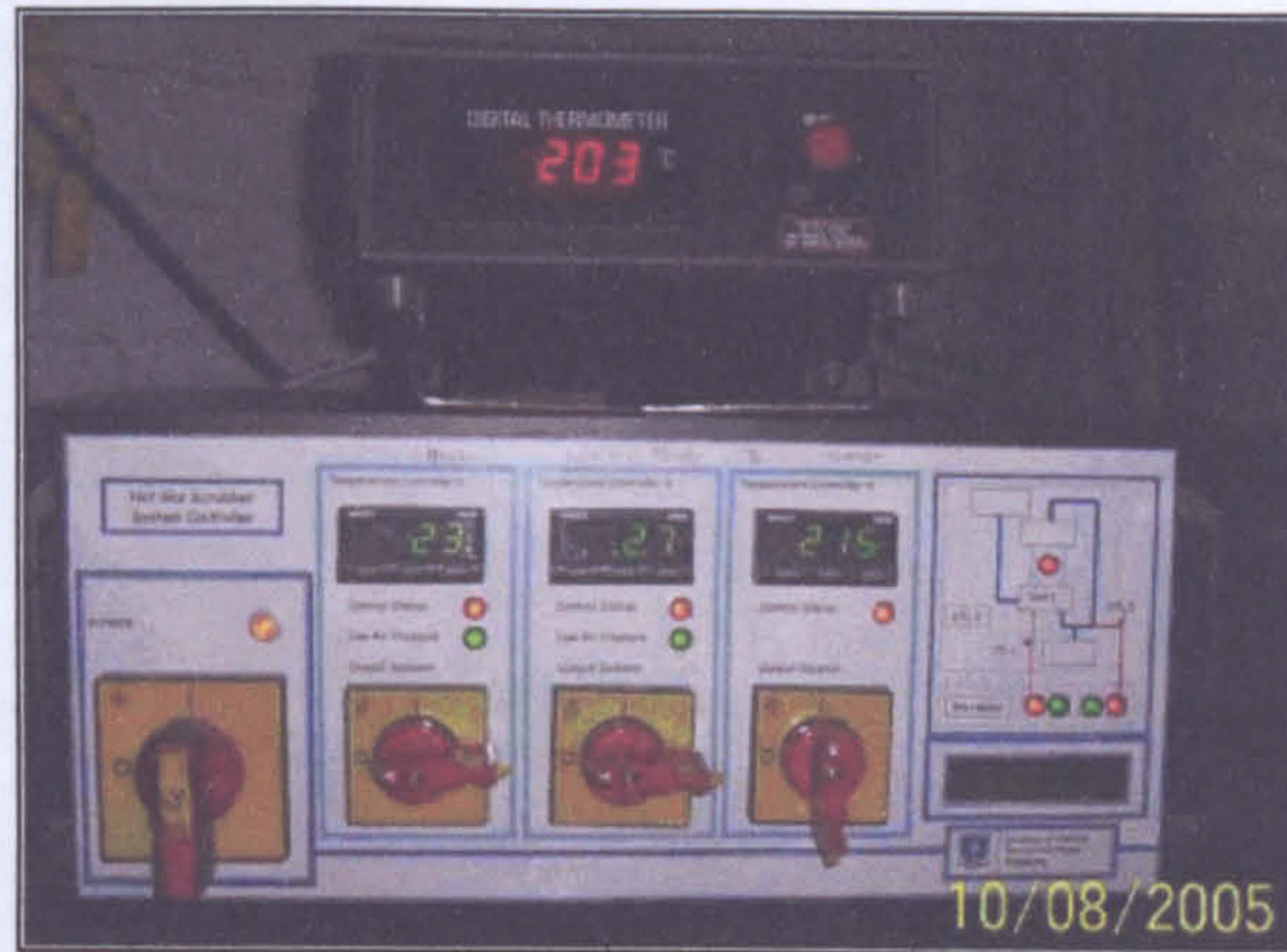
Figure 5.7: Electronic system controller
