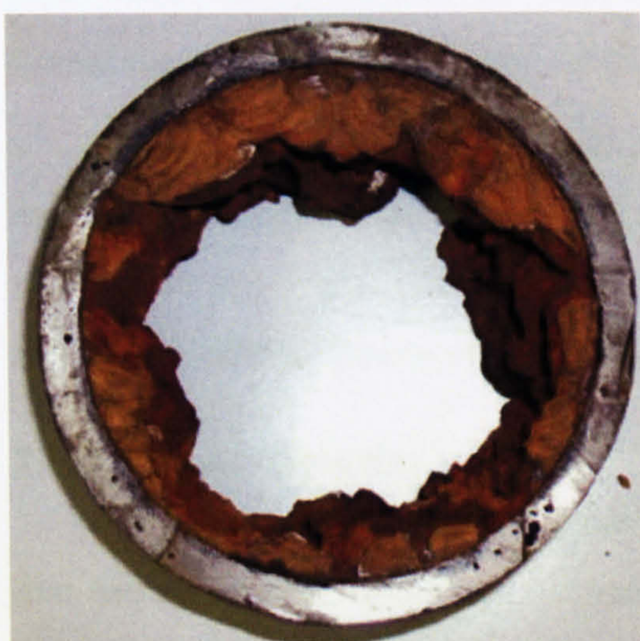
Figure 3 Iron corrosion in a 6' cast iron water main. (www.corrosion-doctors.org)
