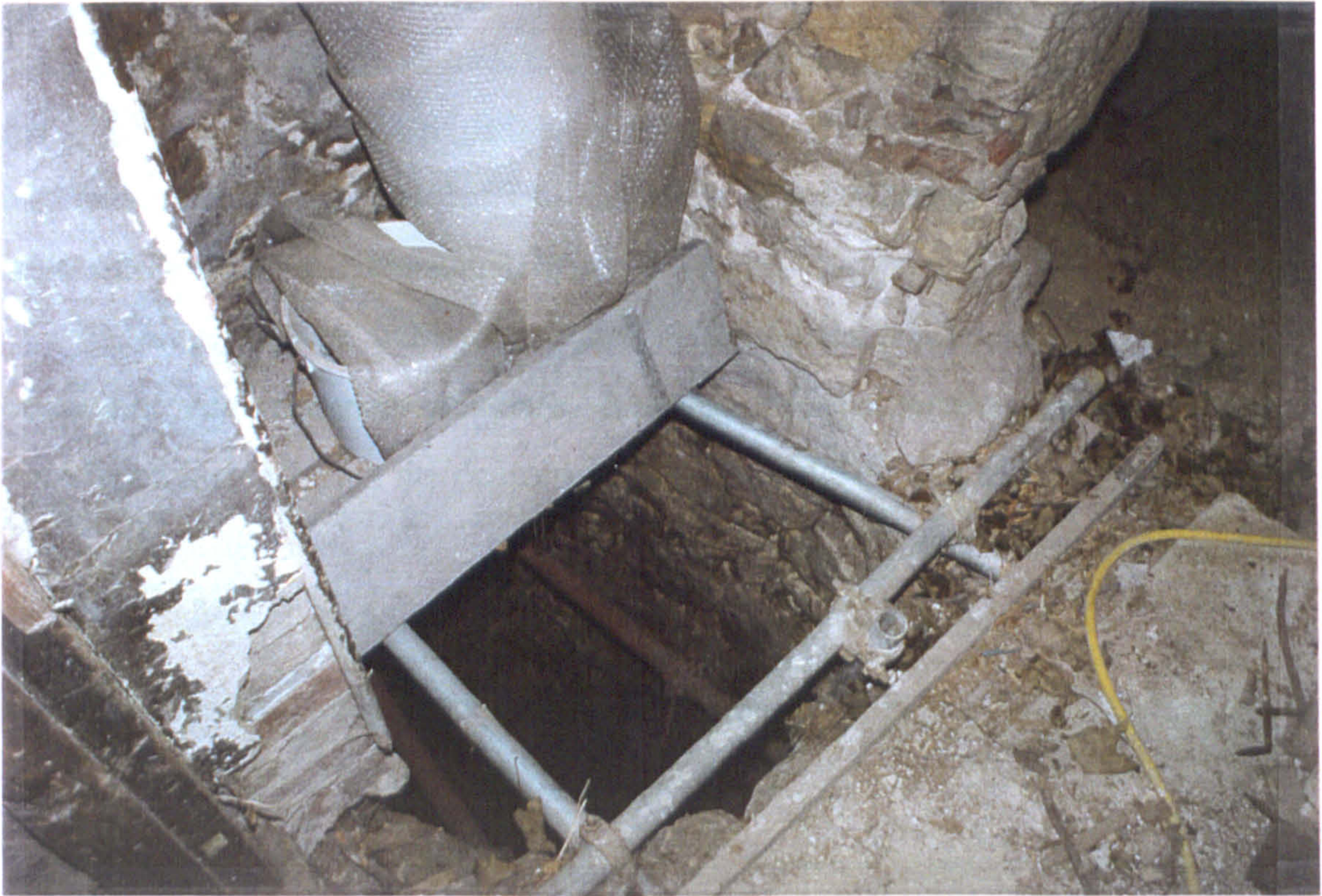
Figure 13. The pit, after excavation, into which waste from the toilet on the floor above would have fallen.
