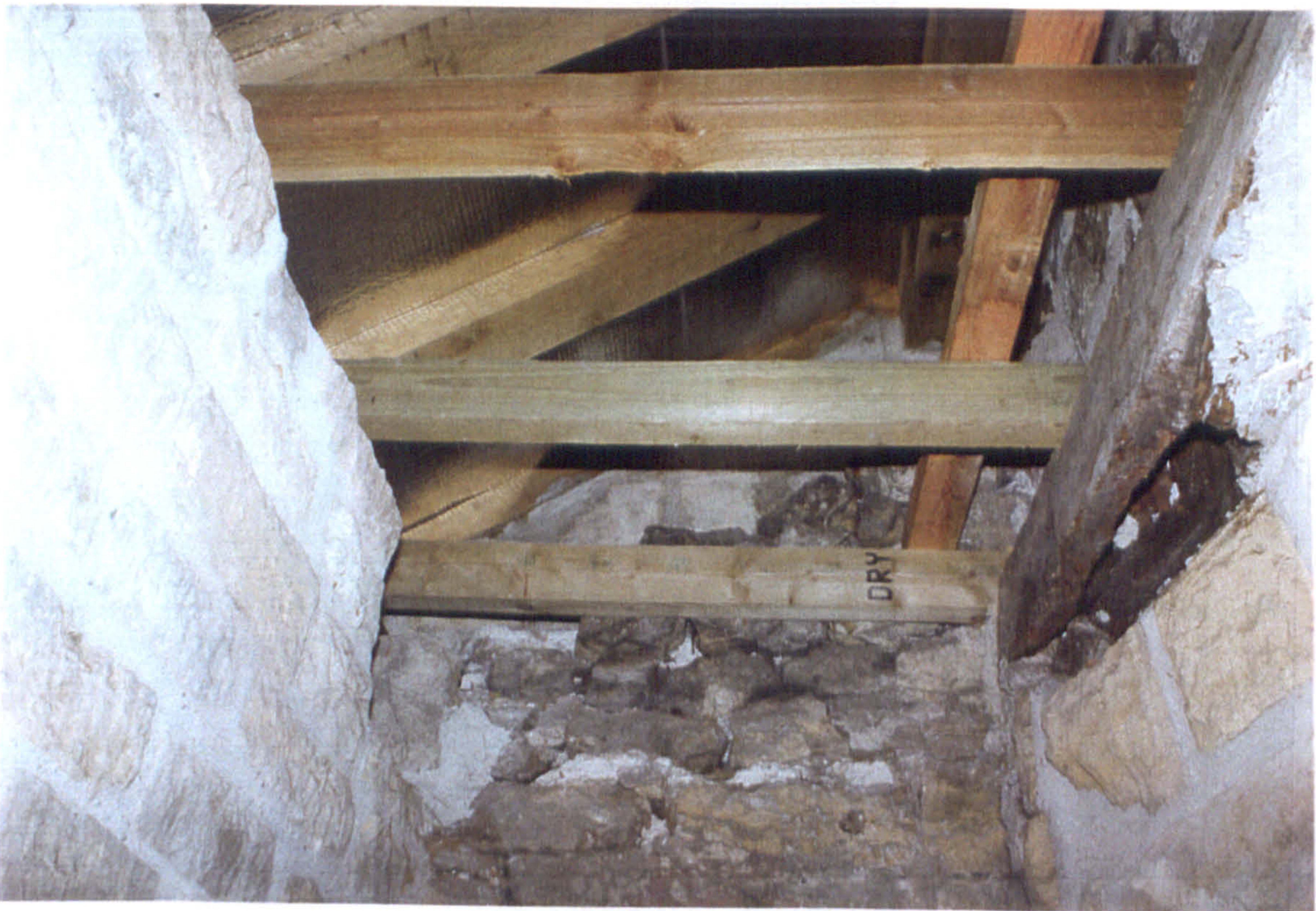
Figure 14. Rafters above the garderobe at Tadcaster, in approximately the same position of those which a roosting owl may have perched.
