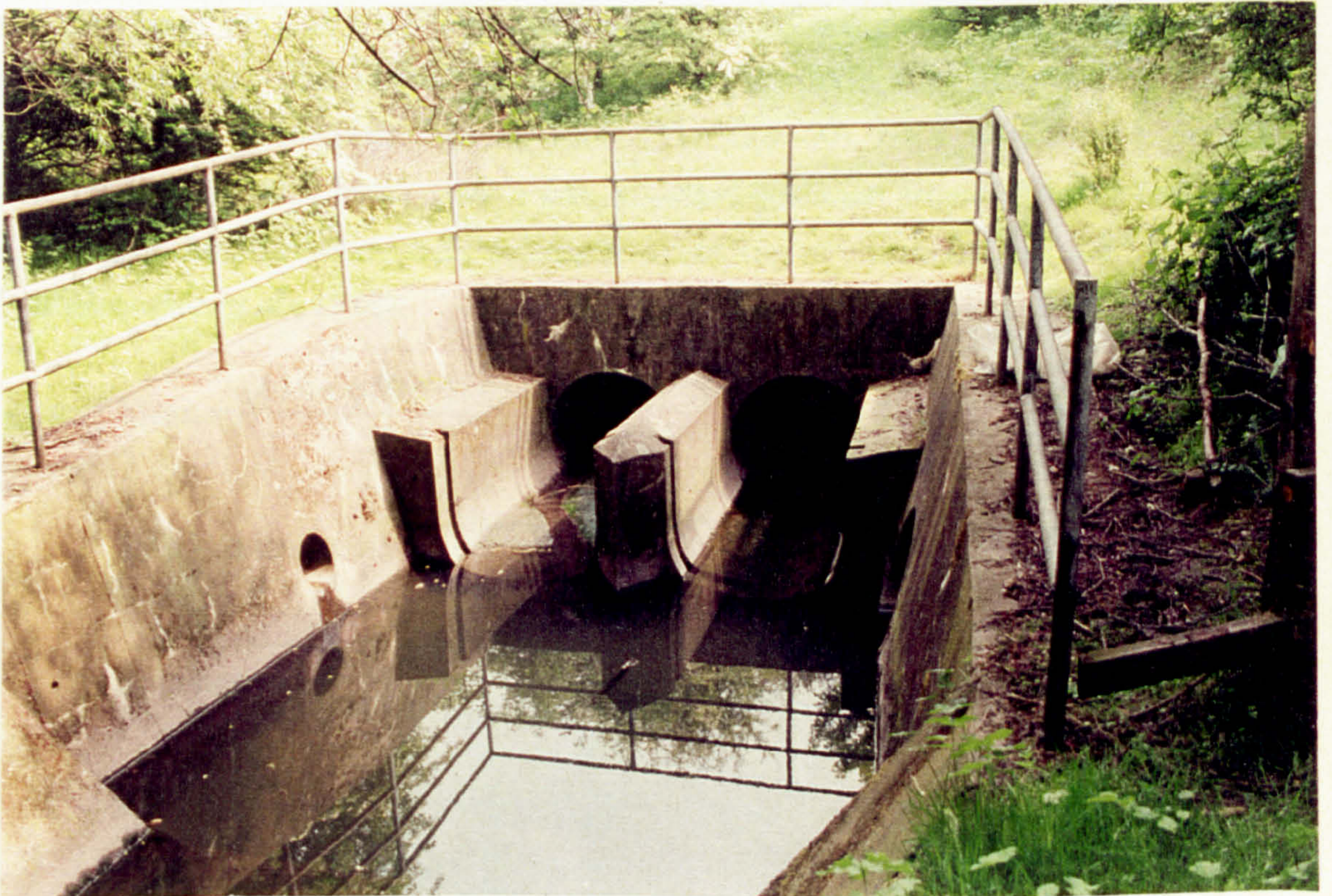
Plate 2.3.d: Pigeon Bridge Brook emerging from beneath the motorway showing the motorway-drainage pipes.
