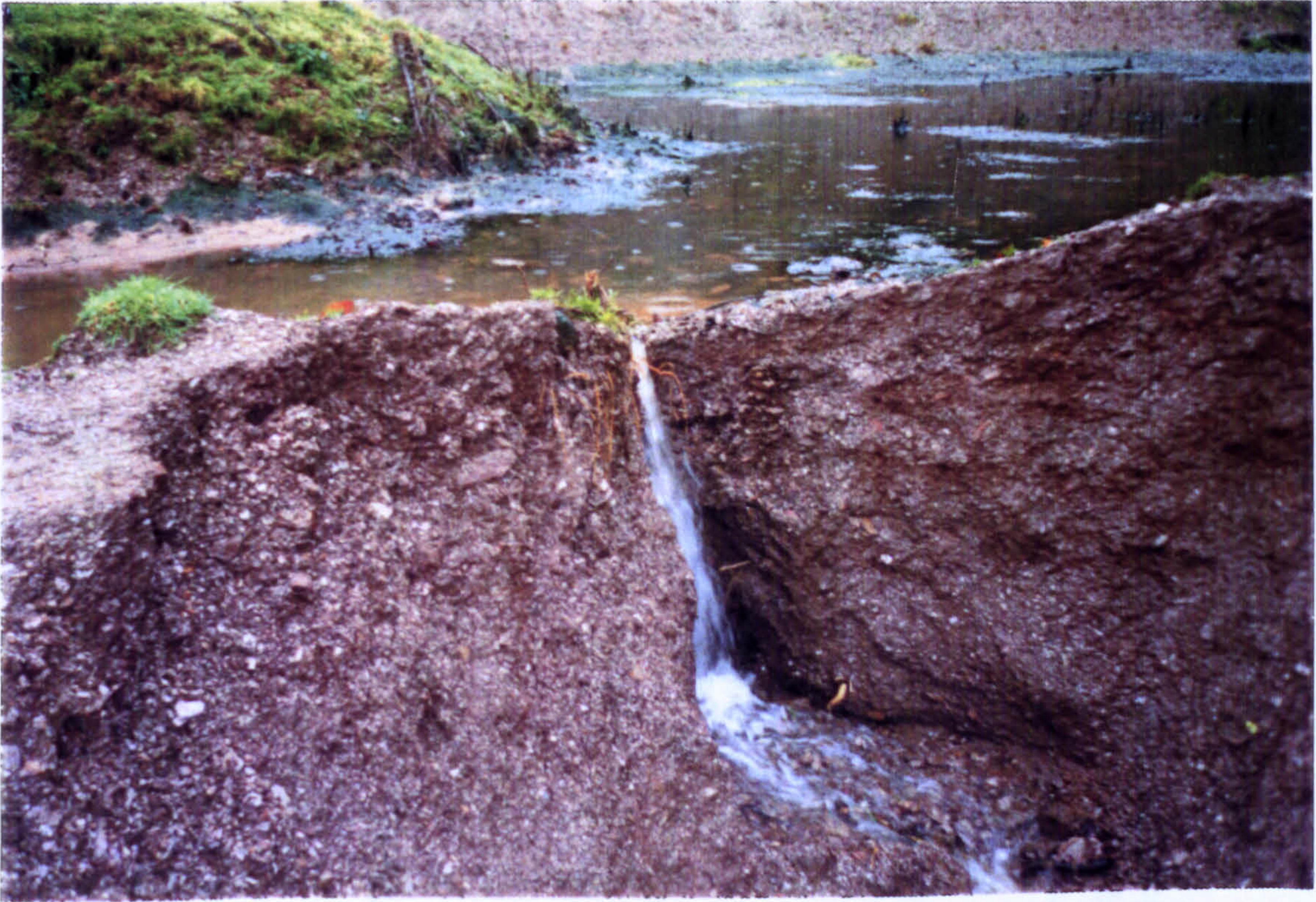
Fig. 4.22. Collapse of the pond retaining bank at Merrifield.
