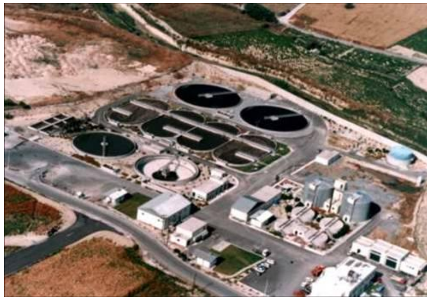
Plate 3.1 Municipal wastewater treatment plant of Heraklion, Greece.
