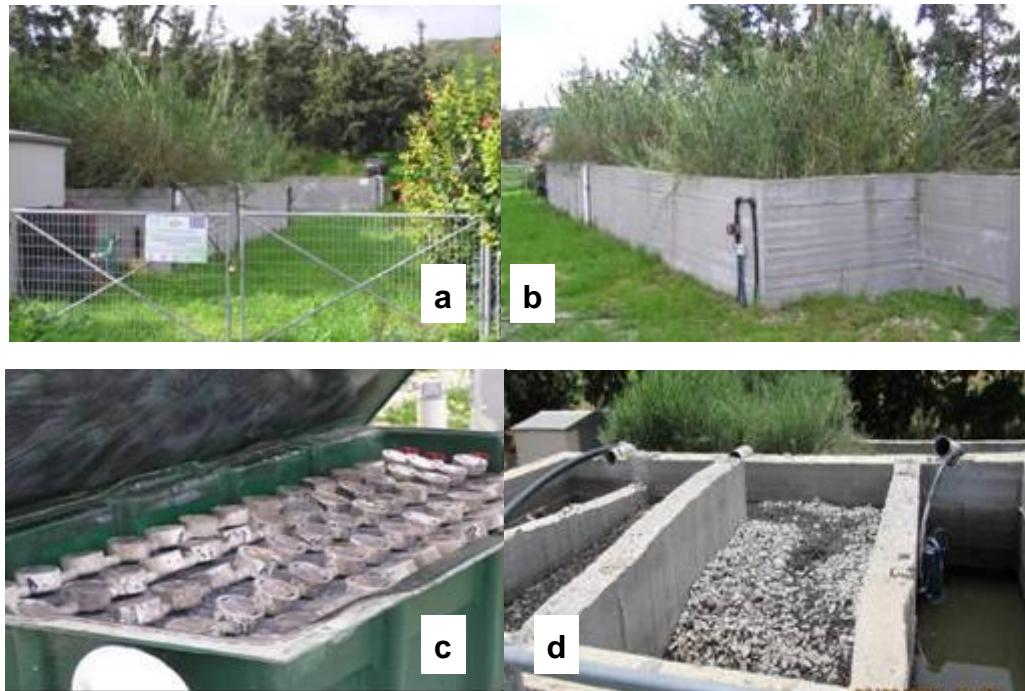
Plate 3.2 Experimental wastewater treatment plant at TEIC, a: general view, b: constructed wetland, c: packed bed filter and d: sand filter.
