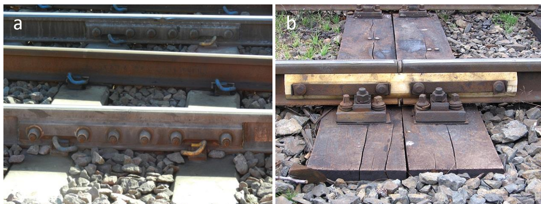
Figure 5: Images showing a suspended joint (a) and a joint supported with two sleepers under the centre of the joint (b) (4)
