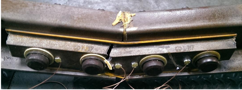
Figure 79: Failure of the standard IBJ due to fishplate failure
