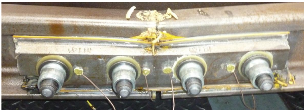
Figure 82: Fishplate of standard rail joint that did not fail due to cracking
