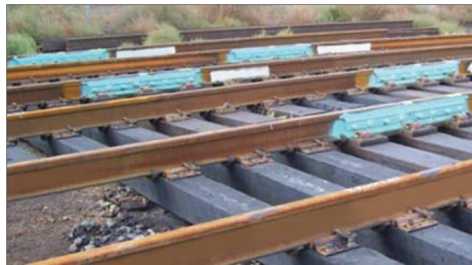
Figure 12: Installed IBJs painted to stop failure by contamination (16)
