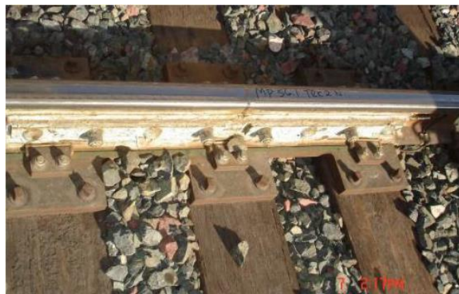
Figure 15: Three sleeper insulated plate used to support the IBJ (3)
