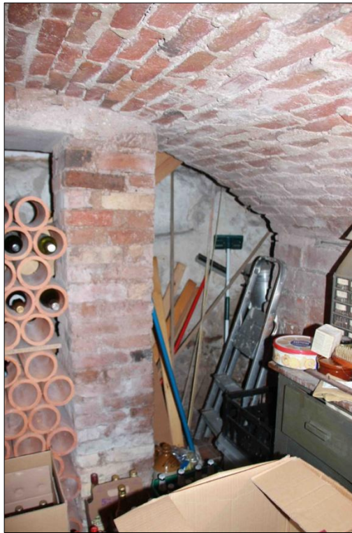
Figure 3.68: Detail of cellar construction at No.16 North Street (source: author's own photo)
