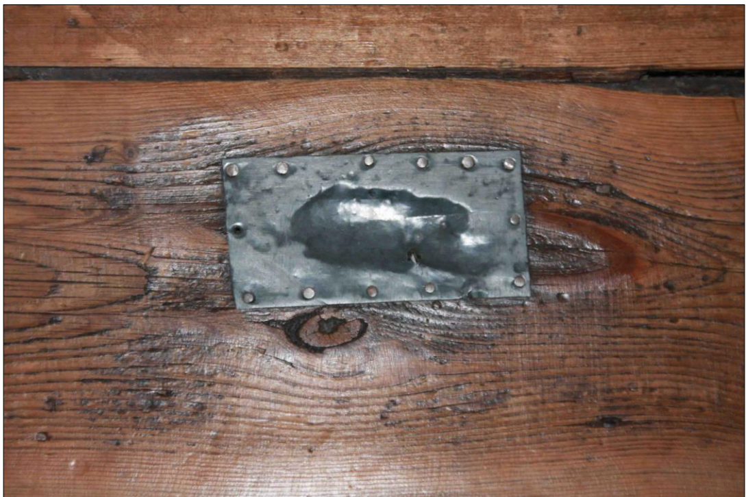
Figure 4.49: Detail of metal repair to first floor of No. 10 Mill Street (source: author's own photo)
