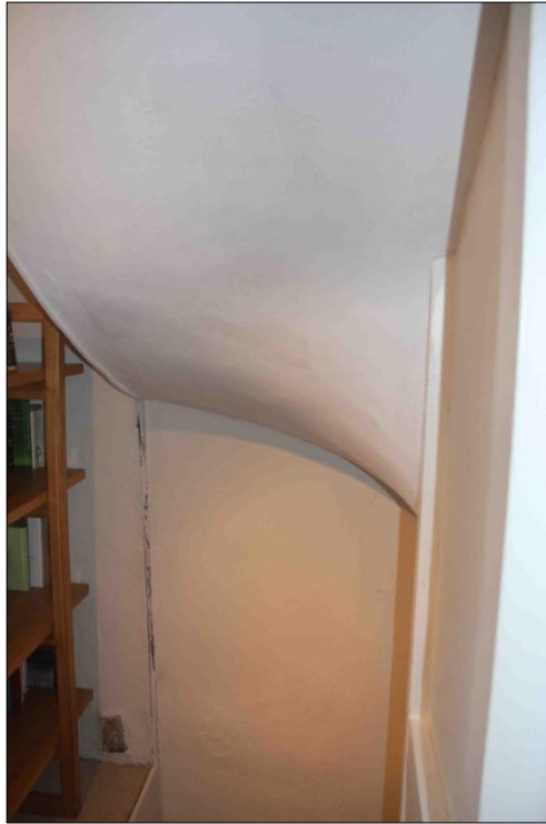
Figure 4.30: Detail of the underside of the staircase of Group I properties (source: author's own photo)
