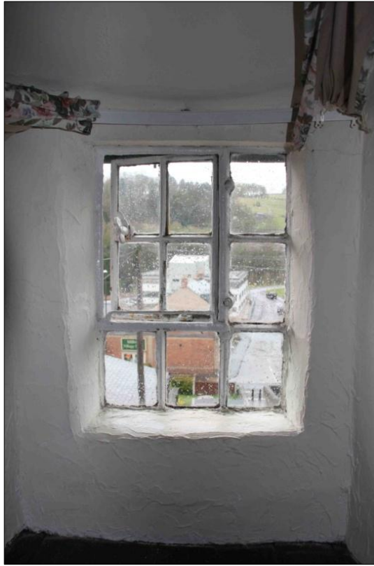
Figure 5.21: Detail of second floor iron-framed window of Group M (a) properties (source: author's own photo)
