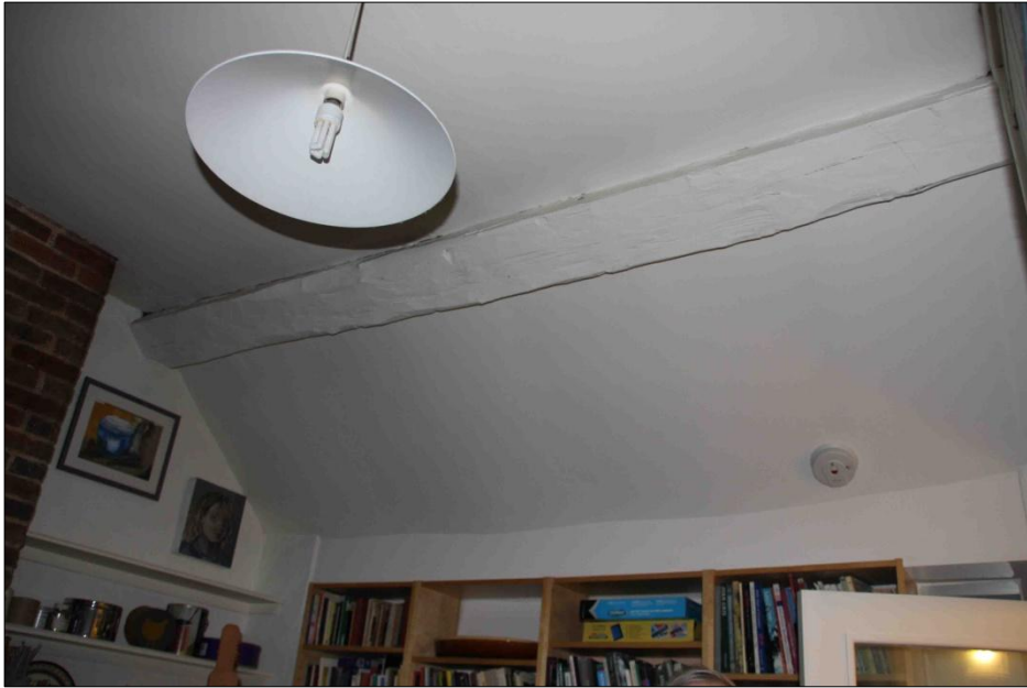
Figure 3.64: Roughly cut purlin at No. 25 North Street, typical within all types of housing at Cromford (source: author's own photo)
