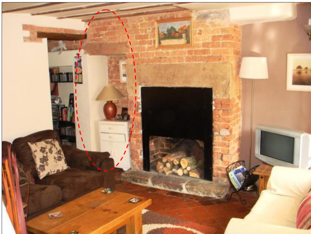
Figure 5.65: Ground floor of No. 63 Hopping Hill, note the recess adjacent to the fireplace (outlined) (source: DCC)
