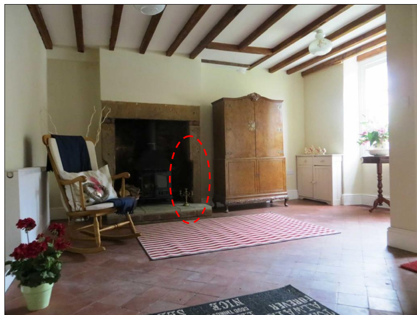
Figure 4.37: Fireplace at No. 30 Long Row, note the modification to the bottom third of the jamb (circled) (source: DCC)
