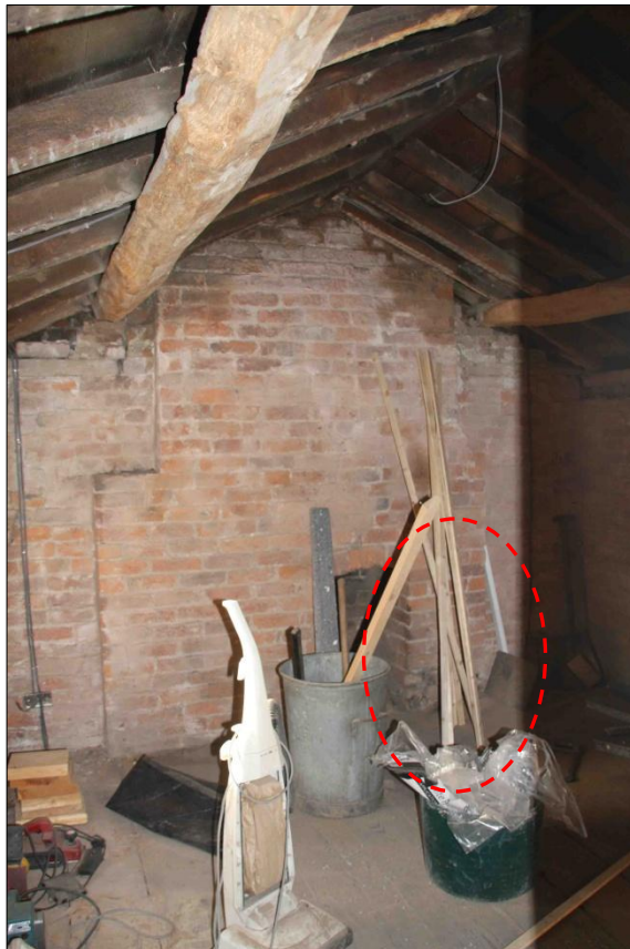
Figure 4.45: Small segmental arched brick fireplace used at Mill Street (source: author's own photo)
