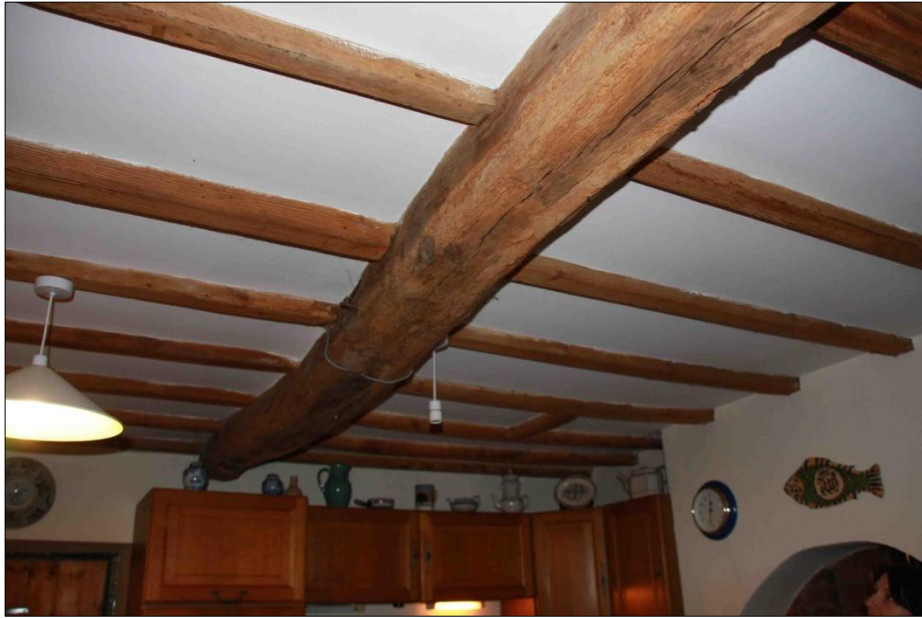
Figure 3.62: Ceiling beam and joists at No. 16 North Street (source: author's own photo)
