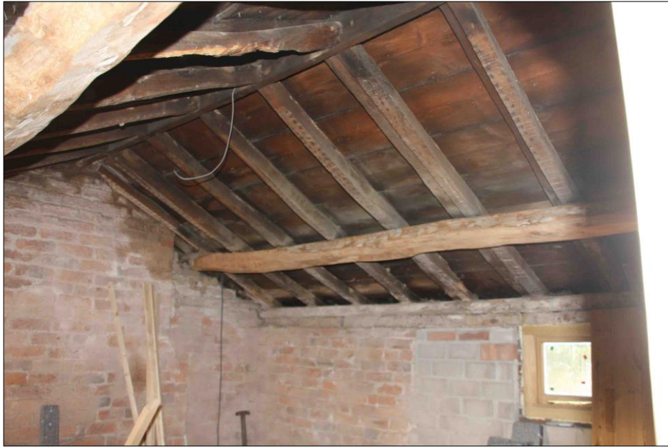
Figure 4.50: Detail of roof structure at No.15 Mill Street (source: author's own photo)
