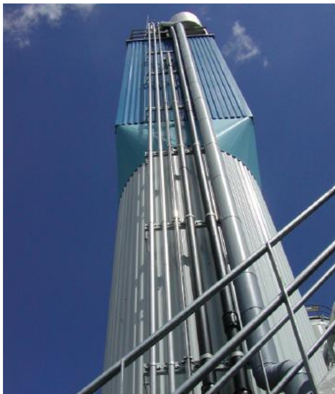
Figure 2.18 Full scale Anammox reactor at Dokhaven STP, The Netherlands Courtesy by Paques
