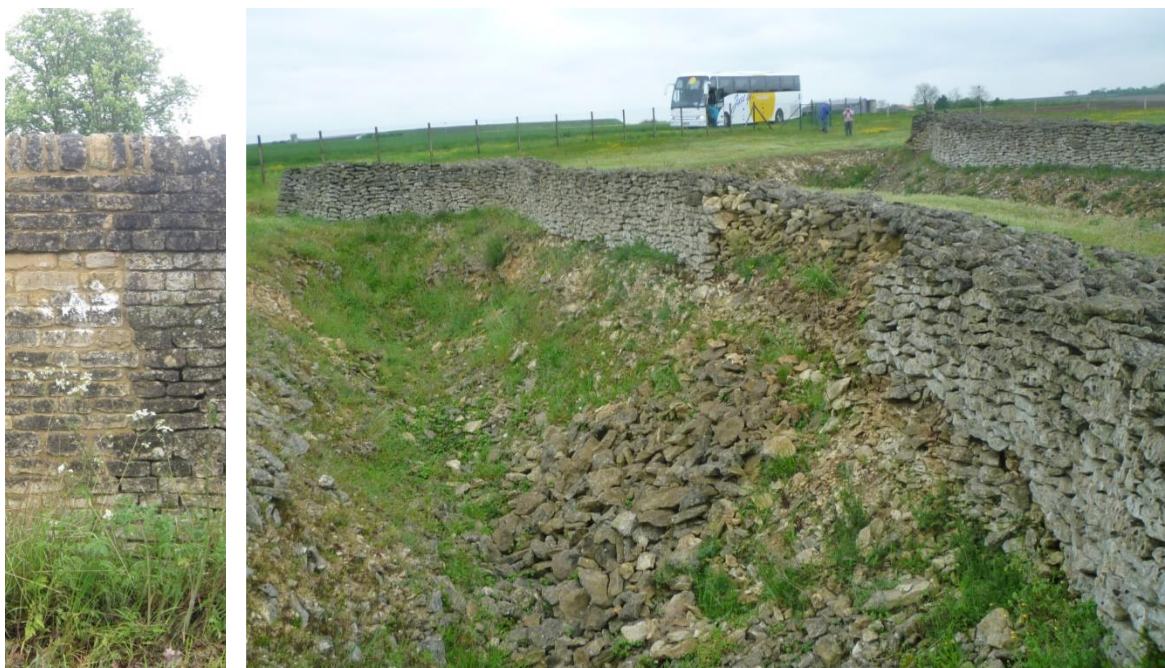
Figure 10.3b: The limestone walls of the enclosure at Champ-Durand in the Vendée of south-west France. Inset left: a Barnack limestone wall, showing the colour difference between fresh and weathered stone.
