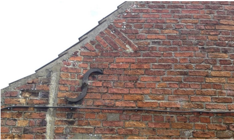
Fig. 10. The Cottage's western gable showing many repairs, but in early brick. Note the straight-line joint with the secondary outshut to the left (rear)
