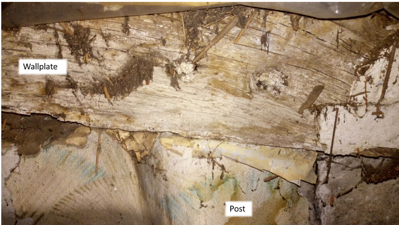
Fig. 32. North-eastern corner of the chamber above the former hall The wallplate is visible, along with the 'now corbel-like', unjewelled post, with double-pegged tenon.
