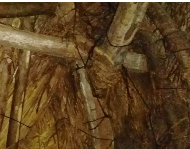
Fig. 49. Enlarged view of principle rafter and collar. Note the nailed-on clasp piece trapping the purlin pole in the angle of the collar, and black string holding on the underthatch and possibly some of the poles
