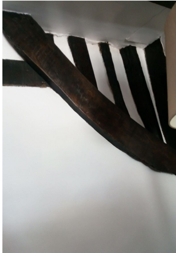
Fig. 58. North-eastern brace in eastern room, with laths exposed from the inside by the current owners. Note also the mid-rail
