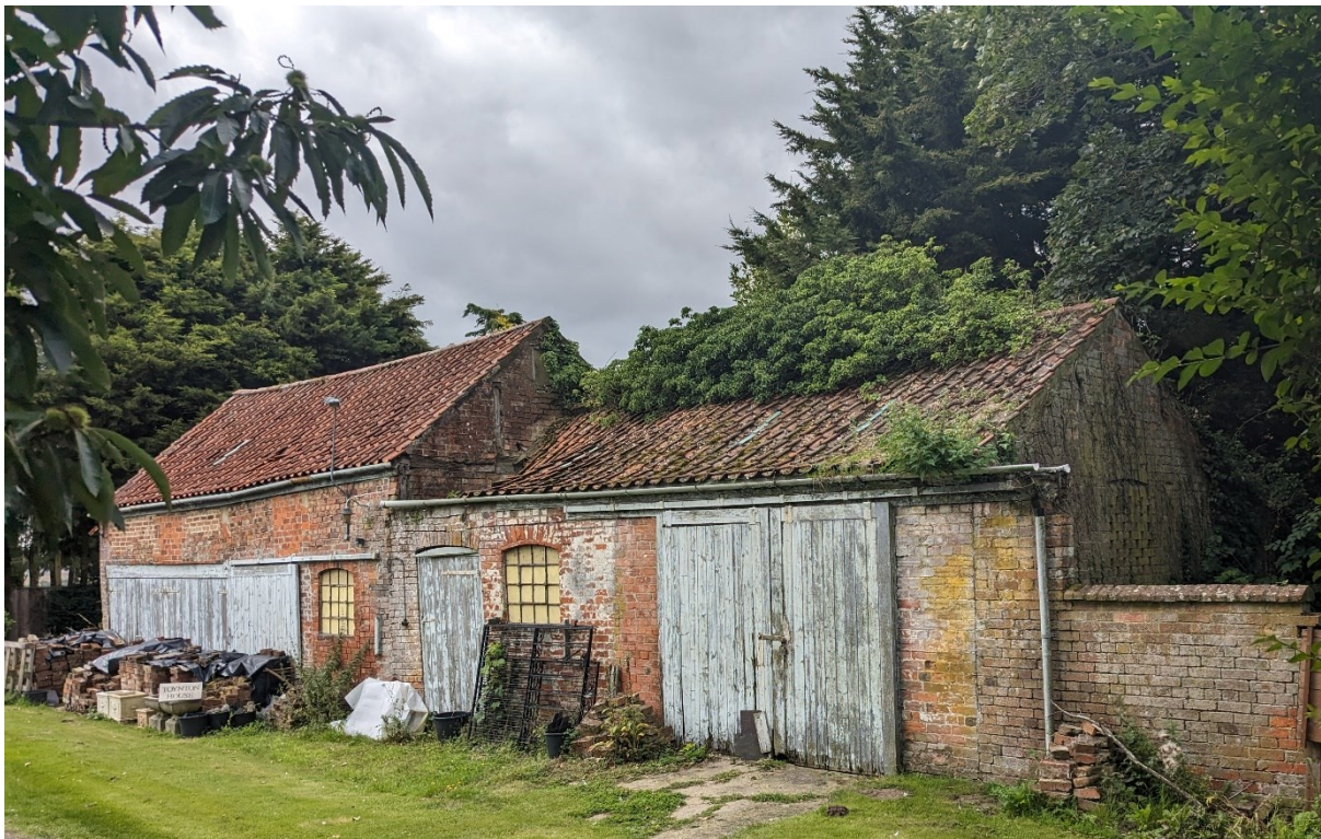
Fig. 128. Toynton House barn. The left-hand, taller part has visible remnants of timber framing in the gable wall
