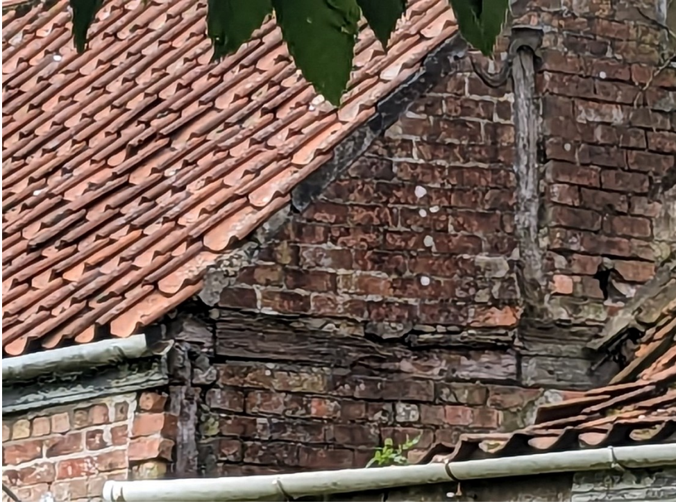
Fig. 129. Close-up of remnant frame. Note the mortise and tenon for the post, and the possibly patched tie beam.
