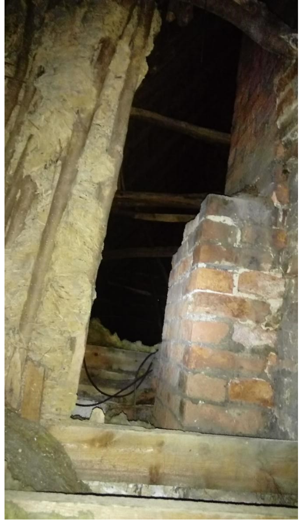
Fig. 50. Looking west from the loft hatch, note the mud and stud partition and later ceiling joists
