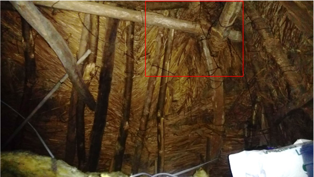
Fig. 48. Roof structure above eastern room, looking north. Note the morticed collar and principal rafter assembly (in red box). The underthatch appears to have been applied at random angles, with an area of darker coloured reeds laid horizontally in the top right hand corner.
