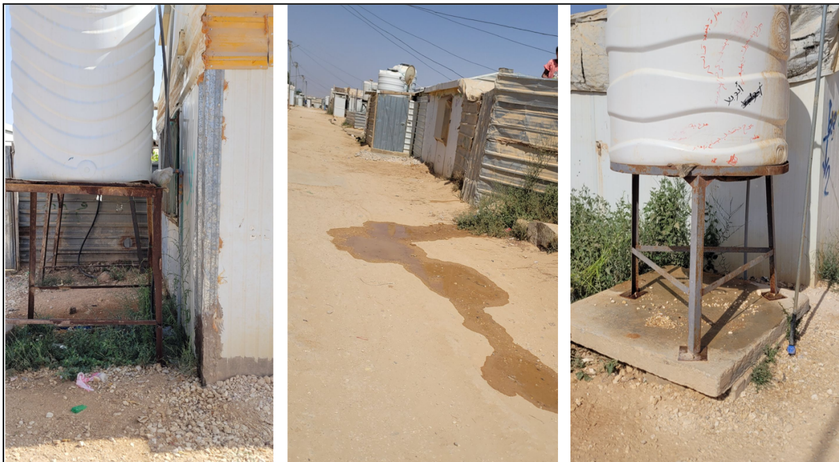
Figure 4.24: Overflowing water tanks lead to water being wasted.
