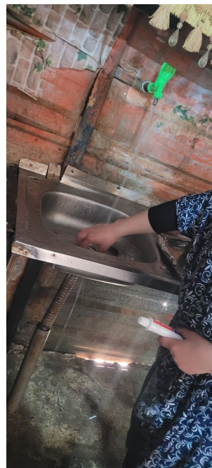
Figure 4.23: Kitchen sink leaking making it inappropriate for toothbrushing.
