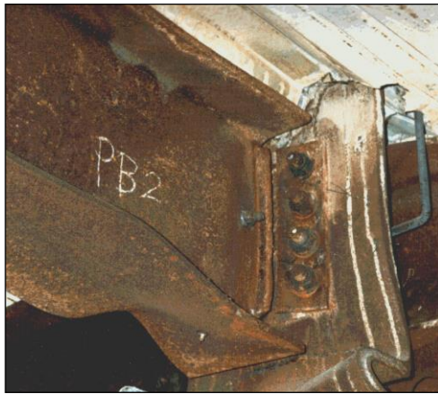
(a) Flexible end-plate connection failure
