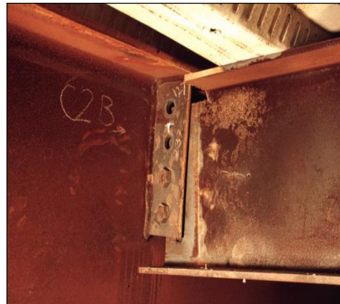
(b) Fin-plate connection failure
