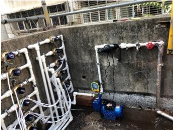
a. overview of valve control unit
