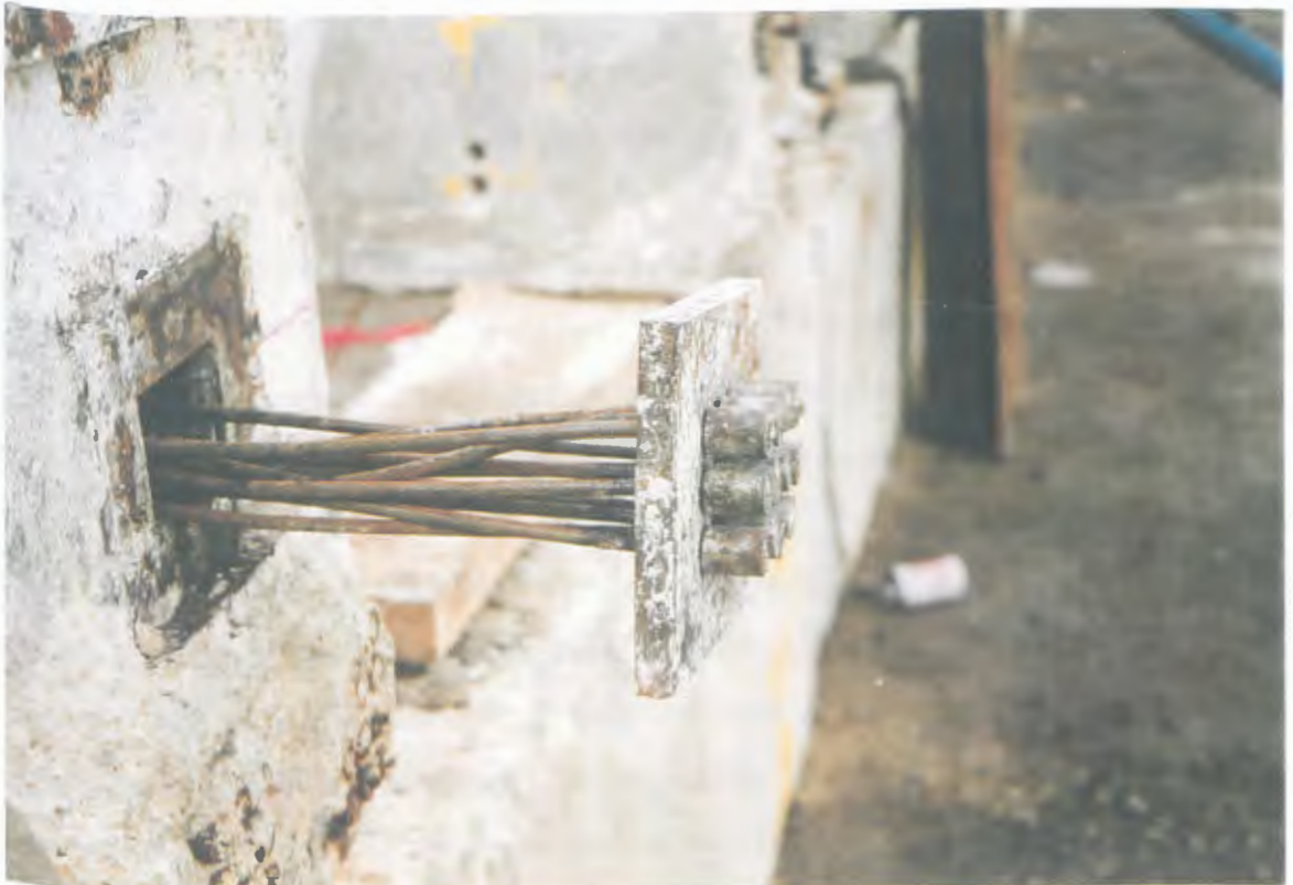
Plate 3.4 Condition at anchorage of one of the Botley beams, showing ungrouted wires
