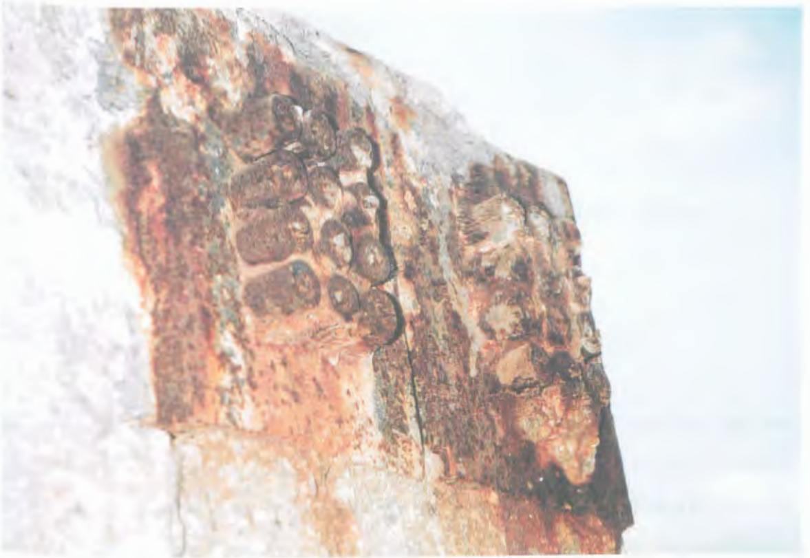
Plate 3.3 Severely corroded collets at the anchorage plate
