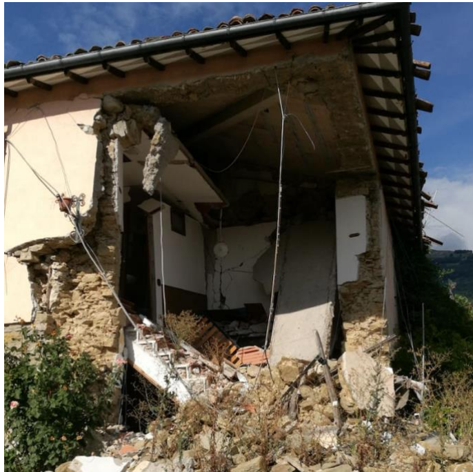
Figure 30: Example of damage caused by the insertion of a concrete ring beam on the roof level (Configno) © Tiziano Palopoli
