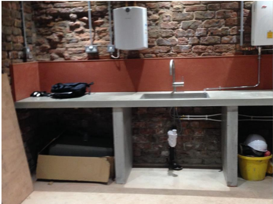
Figure 20: Visit to the building site on the 06-02-2018. New waterproof kitchen installation ©images by the author
