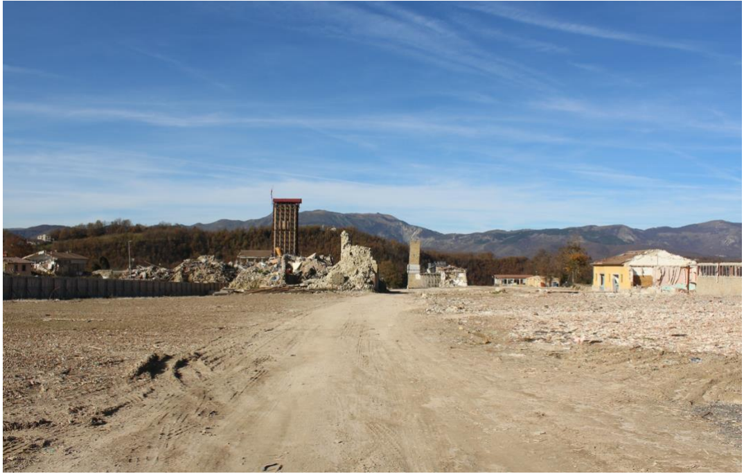
Figure 27: First reconnaissance visit to Amatrice on December 2018. The demolition in the historic centre © image by the author
