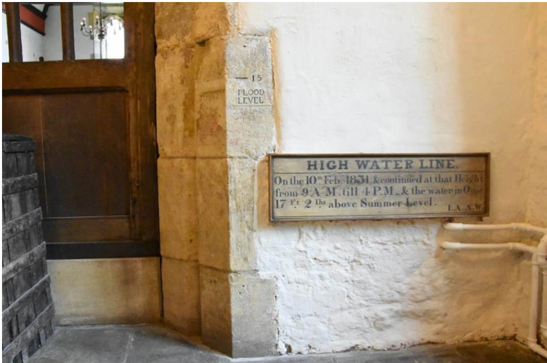
Figure 14: Flood 2015. Flood indicator in the Merchant Adventurers' Hall' ©images by the author
