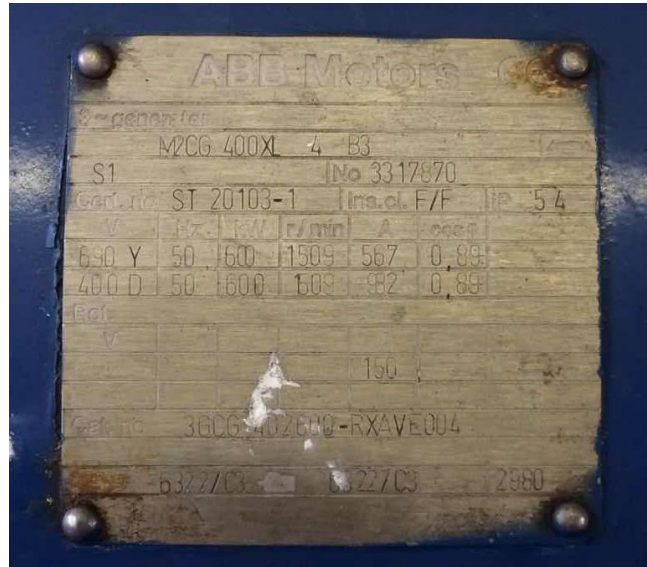
Figure 7.10 – Generator identification plate
