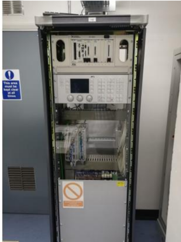
Fig 6. 9 Dynamometer control panel.
