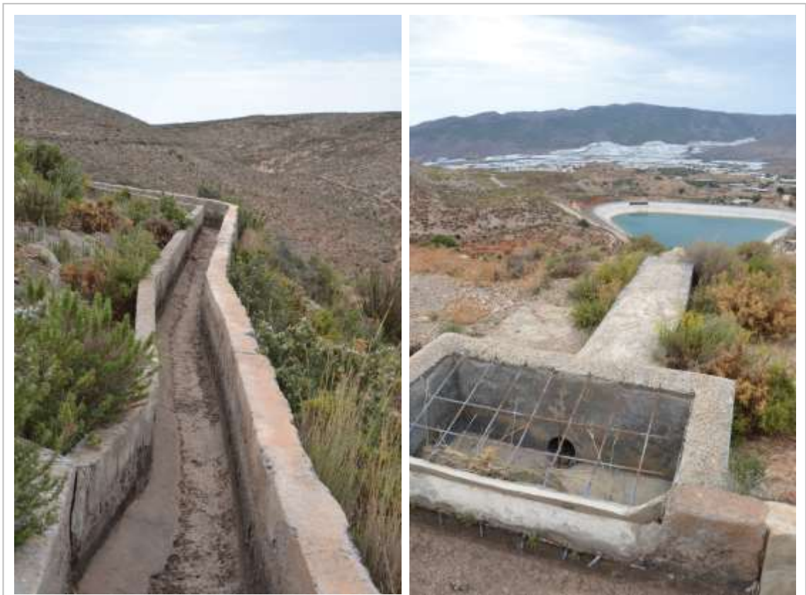
Fig. 3.4. A materialisation of temporal projections in modernisation: the ‘Fuente Nueva’ (literally ‘New Source’) acequia , constructed in Moorish times and modernised through concrete-reinforcement. Once used for the irrigation of terraces, a side-branch redirects to one of a dozen massive distribution basins for greenhouse agriculture. The channel was replaced by plastic tubes in 2010 to increase the ‘capacity to regulate water resources,’ the ‘efficiency in energy consumption,’ ‘water quality control,’ and ‘reliability in distribution,’ and to secure the ‘minimisation of losses’ (SEIASA del Sur y Este 2010), leaving the ‘deteriorated’ channel dry.
