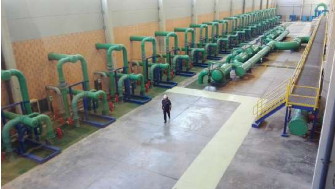
Fig. 3.8. Inside the Carboneras desalination plant: promises of modernisation materialised in pipes, pumps and control systems.
