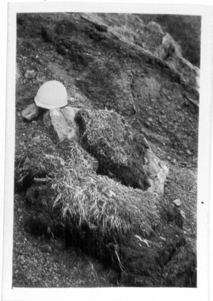
Fig.3-4b Erosion of a riser
