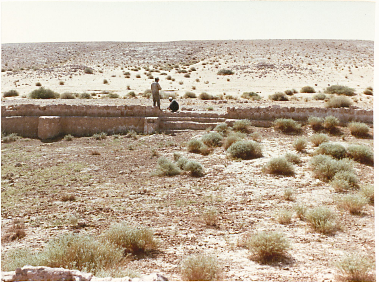
2. Birkat ath-Tha'labīyyah from the west viewing main steps and buttresses in interior.
