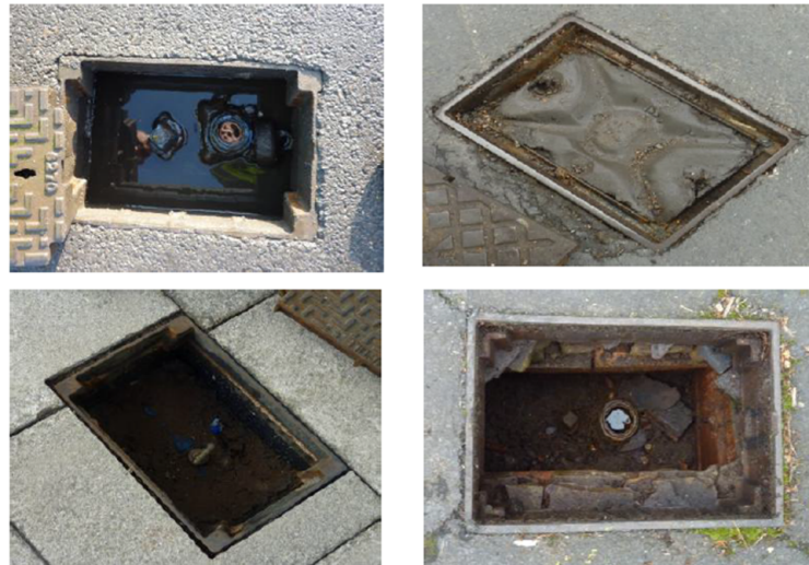
Figure 4.5: Hydrant issues: difficult to access (highways, private premises, loggers fitted), poor conditions (leaks, old, rusty), not present, waste from digging out.
