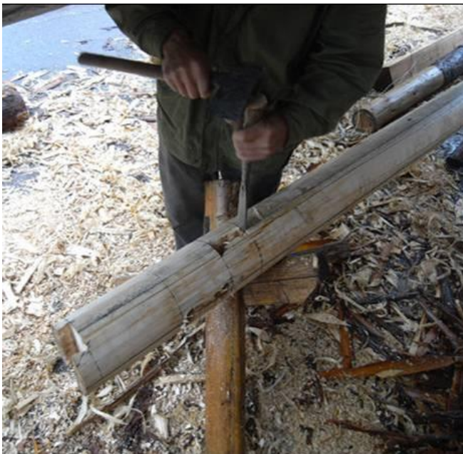
Figure 83. The carpenter Wendong Lu processes the mortises in a tie-beam. Photograph by Derong Kong.
