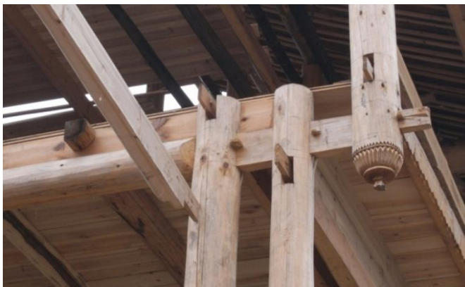
Figure 60. The connecting-tenon, half tenon in a structure, at Xiaohuang village, 2010. Photograph by Derong Kong.
