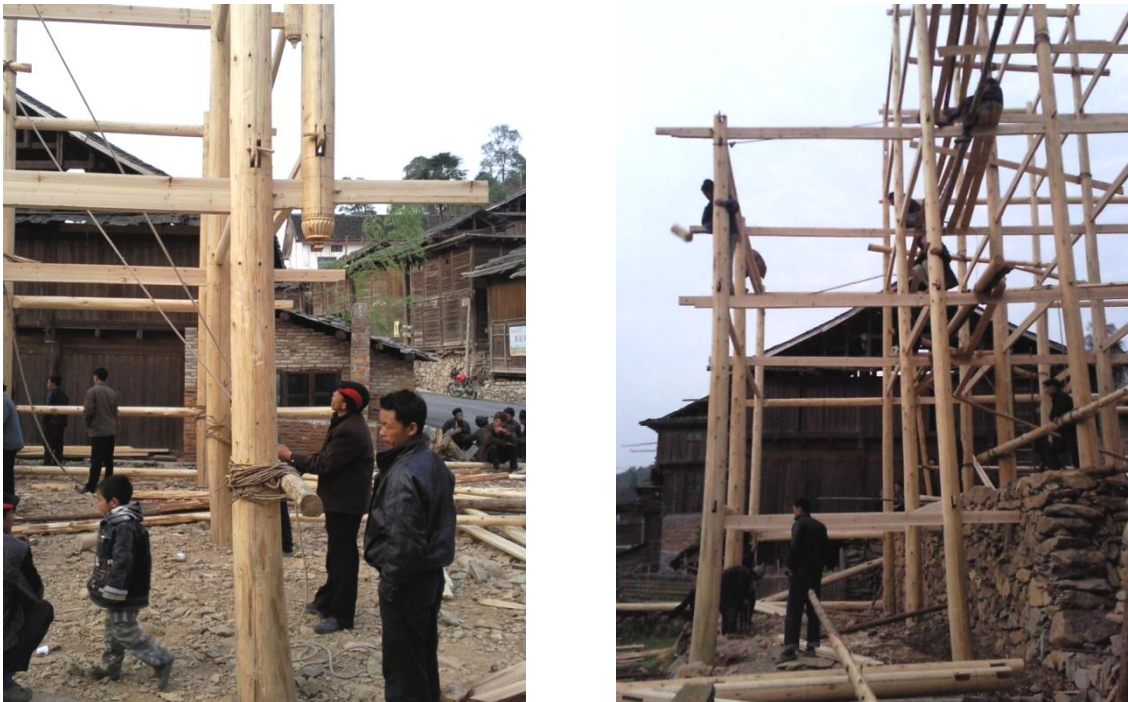
Figure 21. Erecting the structure at Xiaohuang village, in Congjiang County, 2010. Photograph by Derong Kong.
