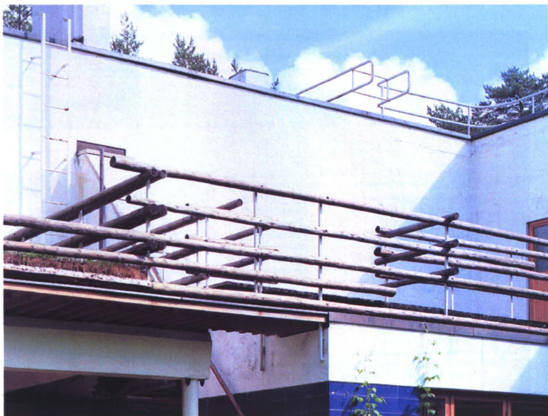
[Fig. 5-84] Balustrade of rustic timber and steel railings on dining room roof
