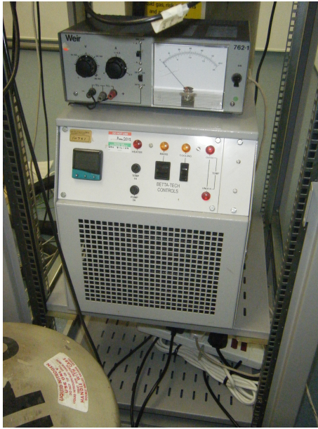
Figure A.4: Heater/Pump used to heat the Insulated Box.
