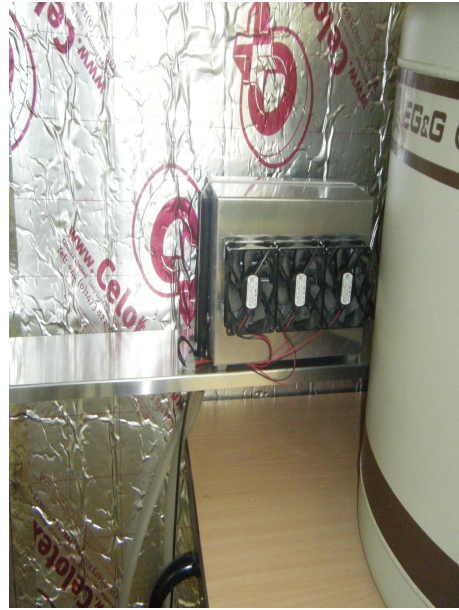
Figure A.5: Fan placed at back end of Insulated Box to circulate the heat.
